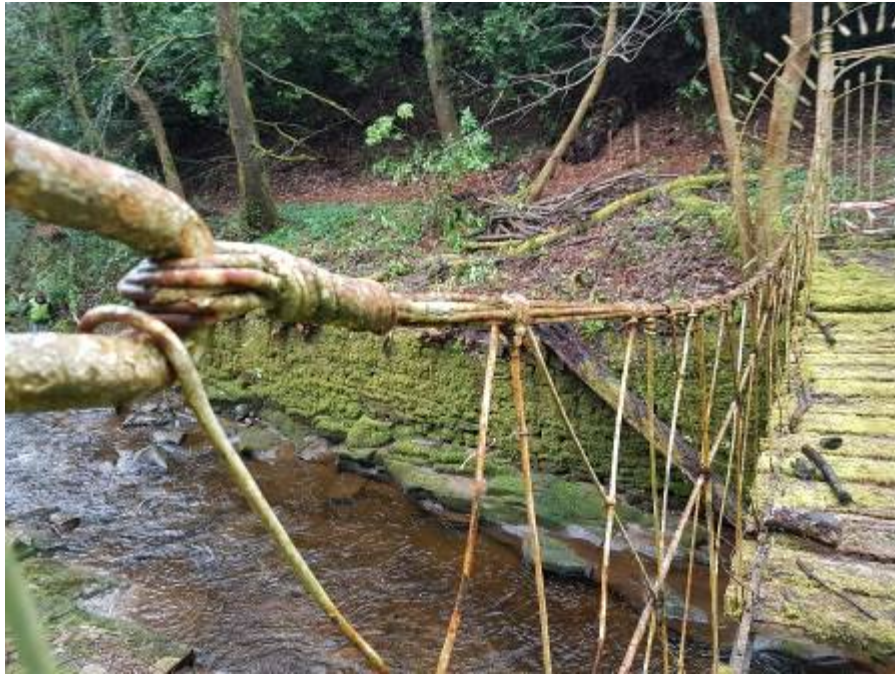
9. Wire cable appears in reasonable condition. Wire hangers are simply wrapped around and bent to suit on site presumably using heat. This is a good sign that they have not cracked or failed during considerable bending.
