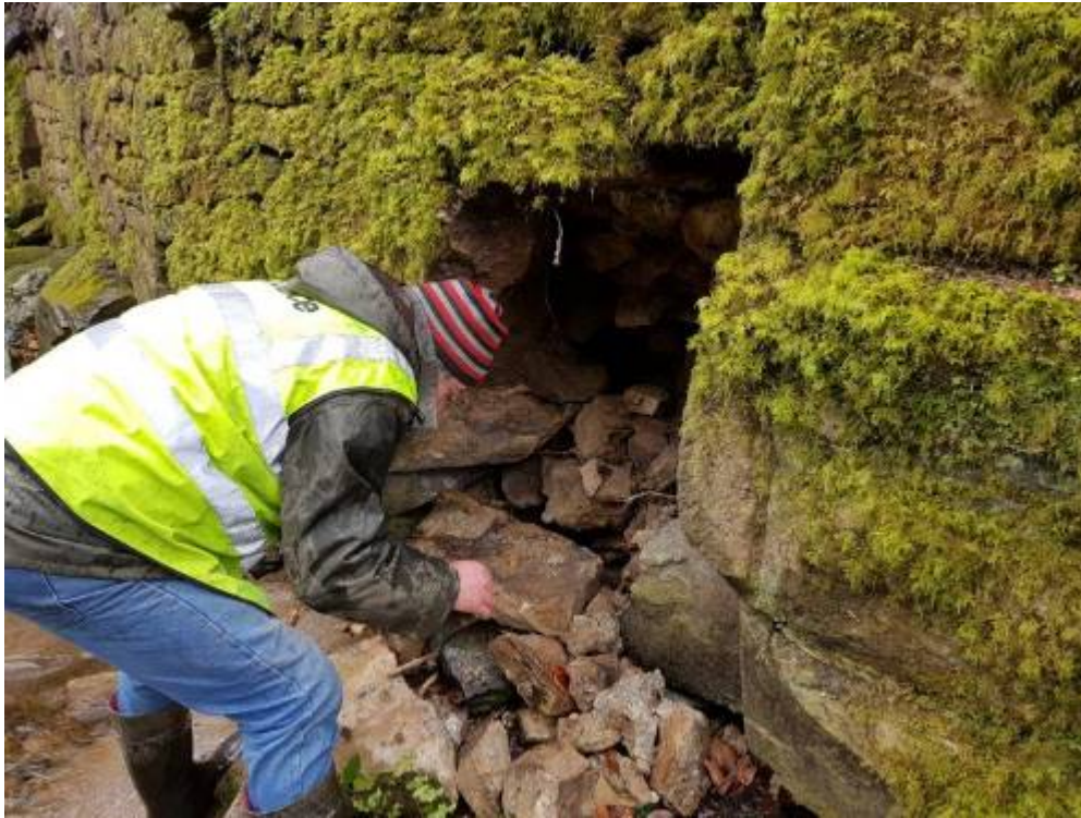
15. Masonry collapse in abutment stonework on Coillte side
