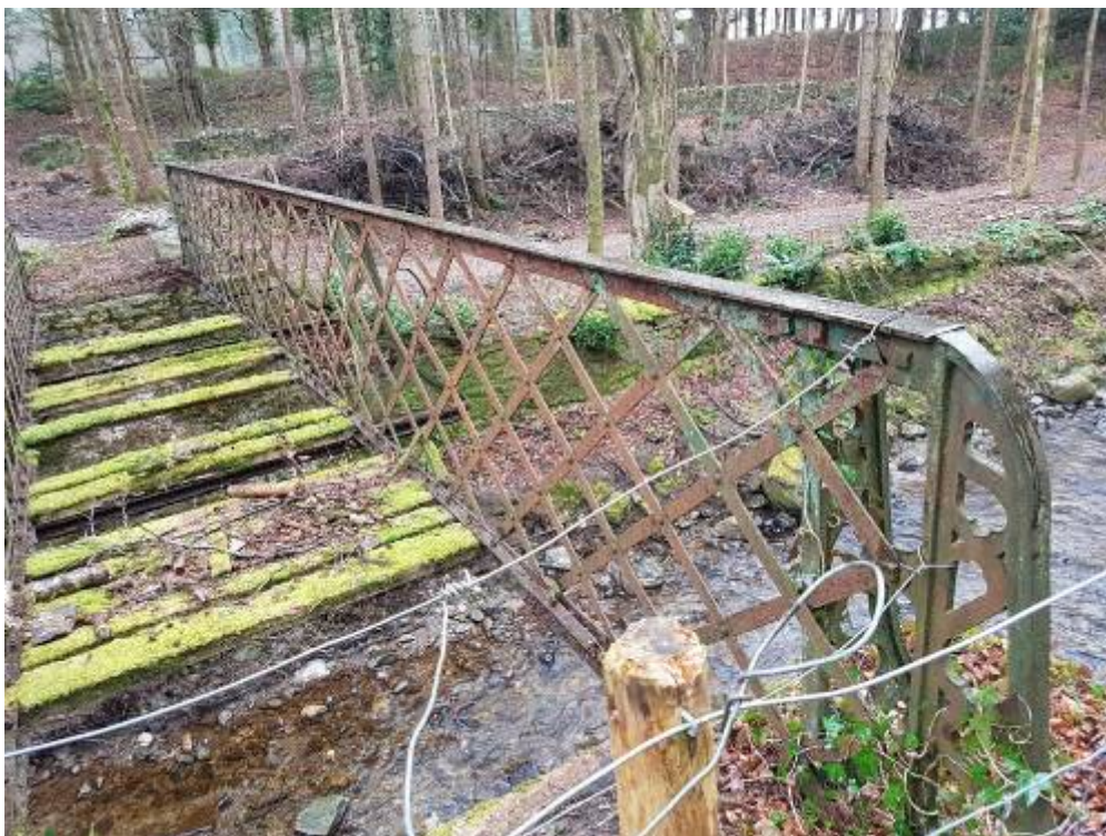
26. General view showing ridge has not deflected in spite of corroded members
