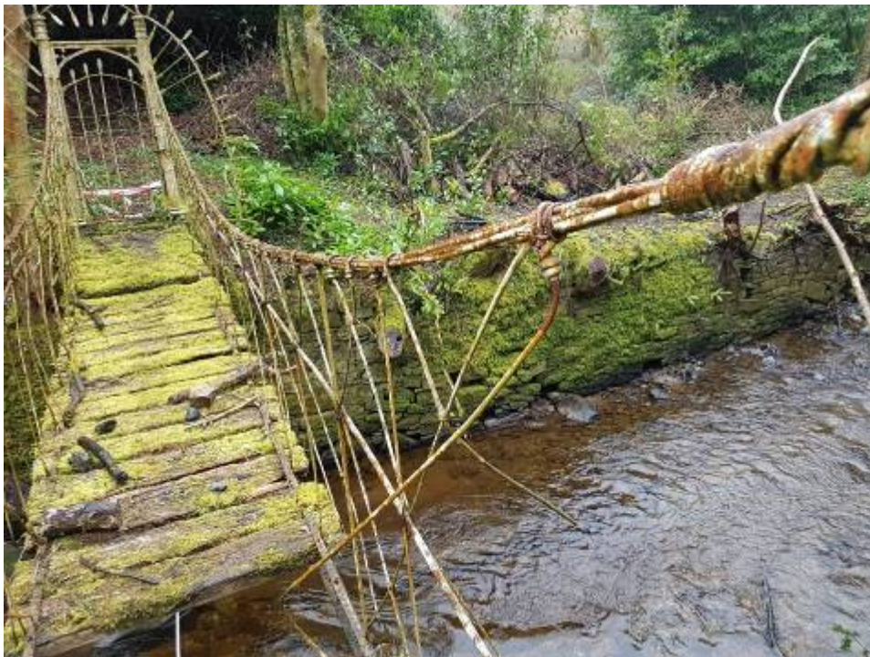
4. Main cable and some missing lattice work
