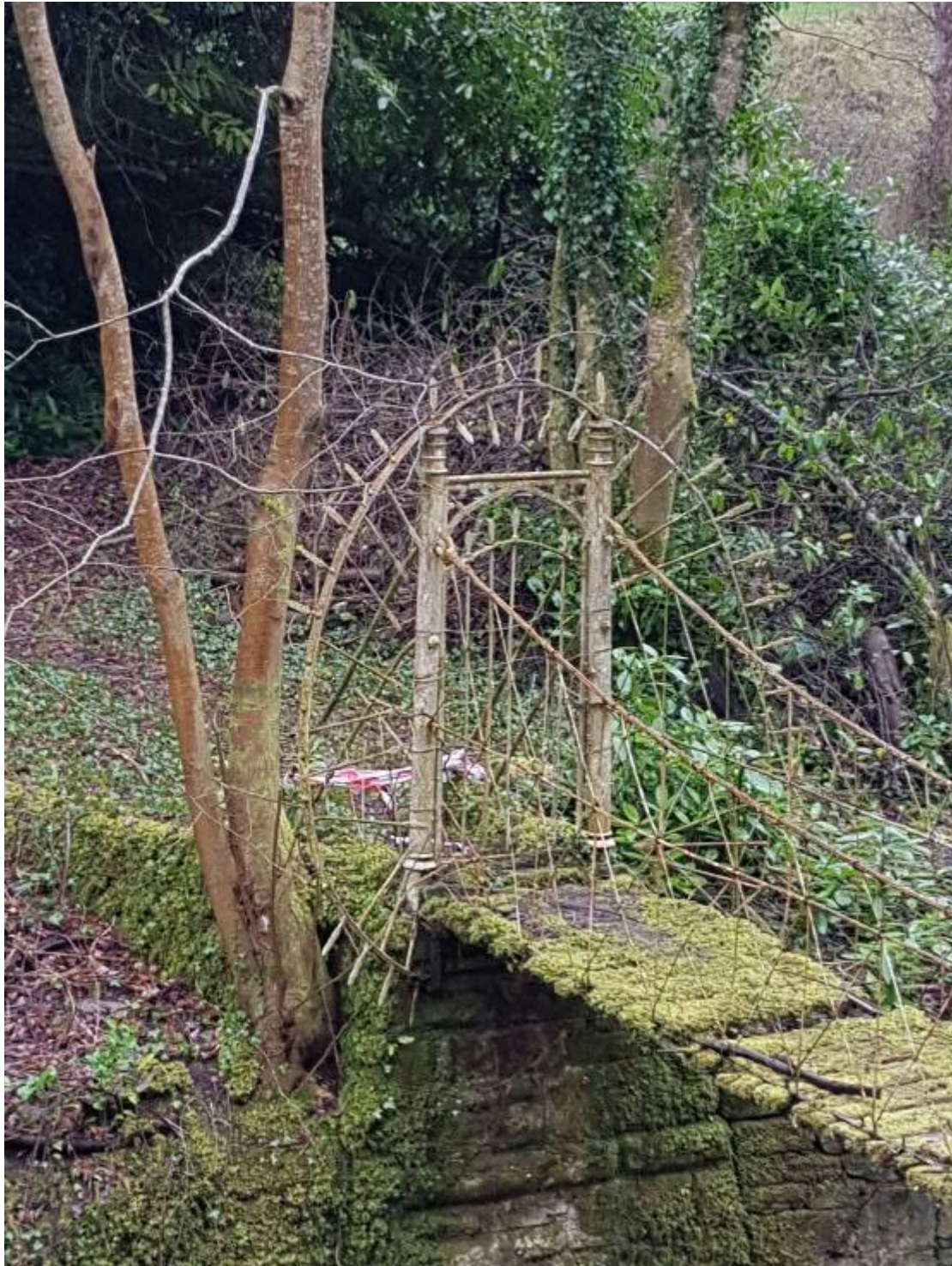
11. The structure on the far side has to be inspected once scaffold is available but appears reasonable
