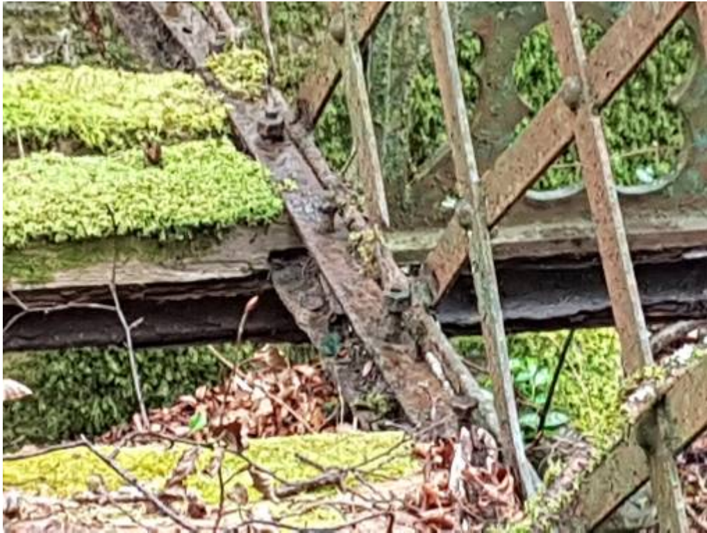
25. 3 cross beams also require complete replacement on a like for like basis. New steel members should be galvanised and etch primed to receive the decorative paint coats
