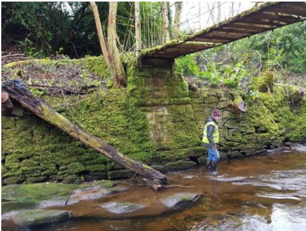
16. Far side stonework requires pointing only
