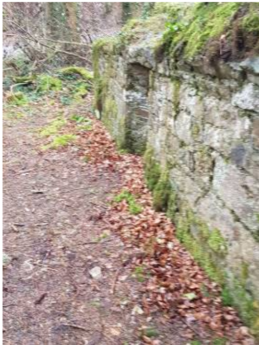
20. The stonework is coursed rubble and dates from the early 19 th century
