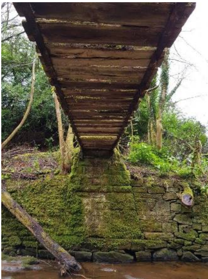
14. Flats appear to be bolted at hanger positions
