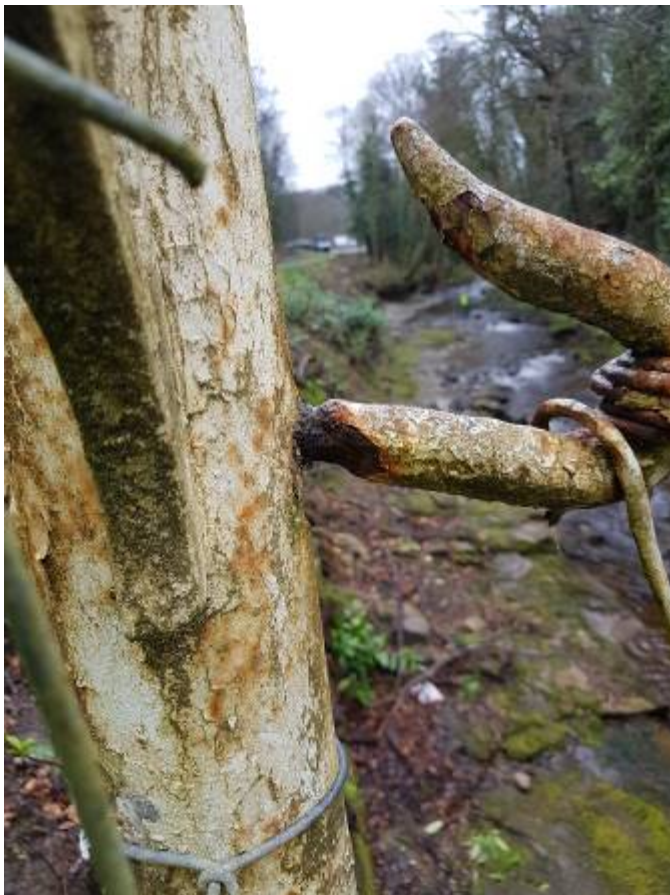
6. Serious corrosion to critical 1 ½ inch tension stays implies replacement
