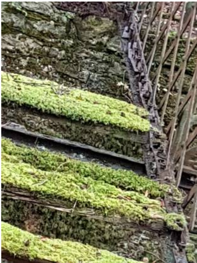
24. The bottom 3-inch x 3-inch angle requires replacement together with the non-structural flat above since water has lodged in the deck area causing extensive corrosion
