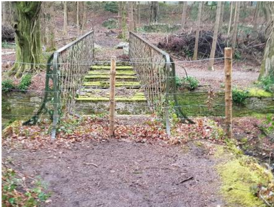
21. The lattice bridge (Bridge 2 ) replaced an earlier bridge and dates to circa 1900
