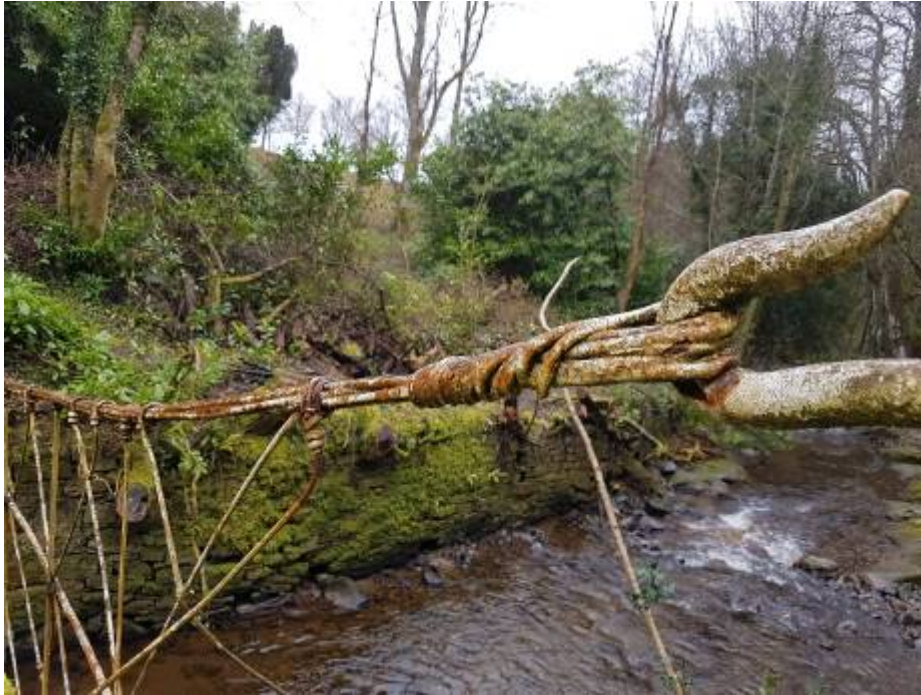
5. Main cable consists of 8 No ¼ inch wrought iron rods and is in reasonable condition
