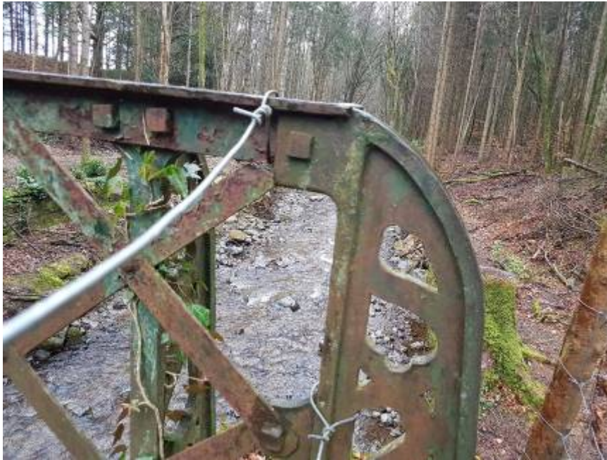
23. A few diagonal lattices require replacement, but the top member is in good condition
