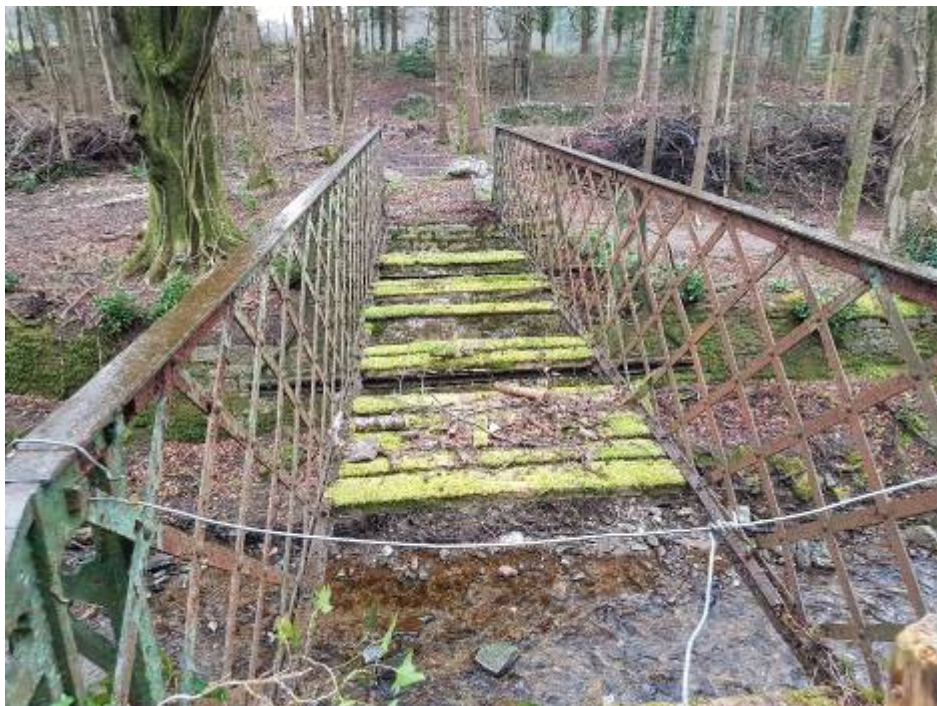
22. Deck required complete replacement
