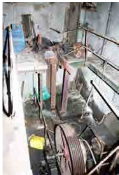
OFIAR-008-038_11 FWH 15/10/2003 Generator in boiler/generator house.
