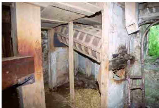
OFIAR-043-002_12 FWH 18/07/2003 Mill: inclined shelling stone rotary sieve on ground floor of east bay.
