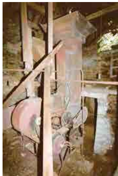
OFIAR-009-006_14 FWH 11/06/2003 Kiln: oil-fired dryer in left-hand kiln.
