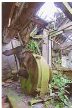
OFIAR-017-036_11 FWH 16/07/2003 Building 2: hammer mill on second floor.
