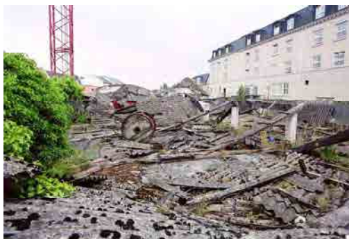
OFIAR-017-064_07 FWH 16/07/2003 Looking east over collapsed roof of malt house.
