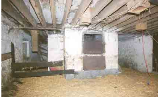
OFIAR-031-012_10 FWH 31/07/2003 First floor of kiln. Note timber-lined walls and brick duct (at left).
