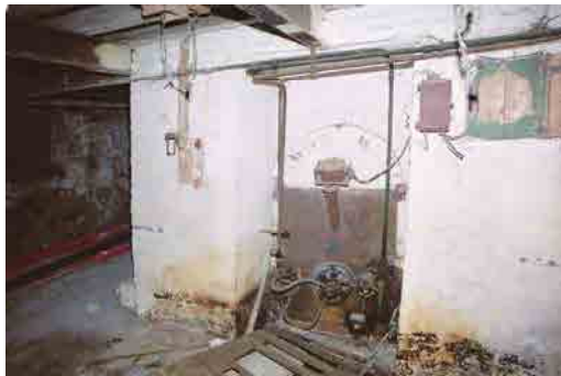
OFIAR-017-064_11 FWH 16/07/2003 Oil-fired furnace on ground floor of malt kiln.
