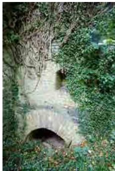
OFIAR-035-034_08 FWH 12/09/2003 Base of chimney abutting north side of north block, from east.
