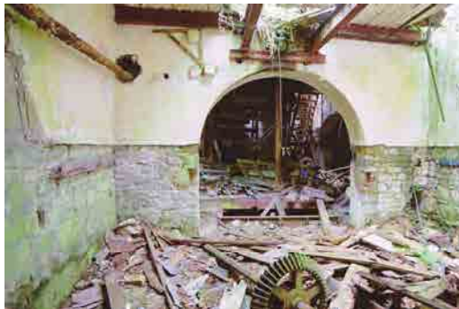
OFIAR-017-036_14 FWH 16/07/2003 Building 3: internal view of ground floor, looking SW to building 2.
