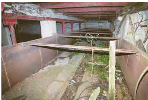
OFIAR-017-064_08 FWH 16/07/2003 Steep tank at east end of first floor of malt house.
