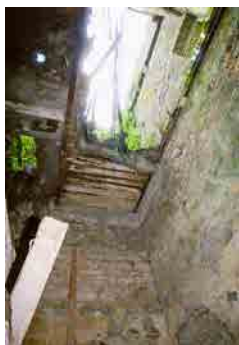
OFIAR-031-005_08 FWH 01/08/2003 Looking up through floors of kiln in north-east corner of mill.
