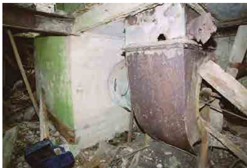
OFIAR-031-005_09 FWH 01/08/2003 Furnace and fan on ground floor of kiln in mill.
