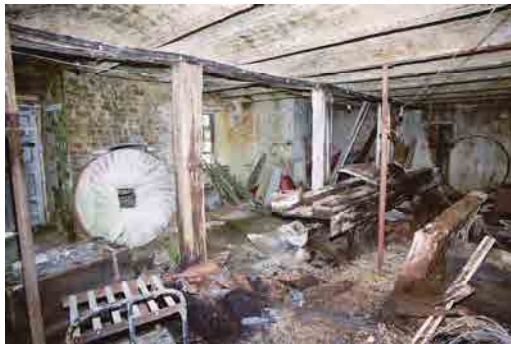
OFIAR-014-004_21 FWH 24/06/2003 Ground floor of kiln, from north-west. Note brick fireholes along wall.
