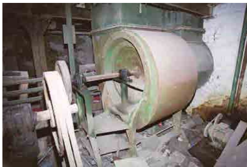
OFIAR-017-064_12 FWH 16/07/2003 Electrical blower fan on ground floor of malt kiln.
