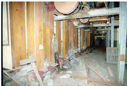
OFIAR-008-038_24 FWH 15/10/2003 Elevators on ground floor of east section of mill, looking north.
