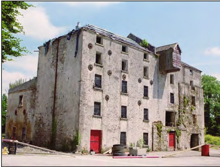
Fig 7.11 Plastic sheeting was nailed to the deteriorated roof of this corn mill at Belmont to prevent further rotting of the top floor and its machinery (014-004.1).
