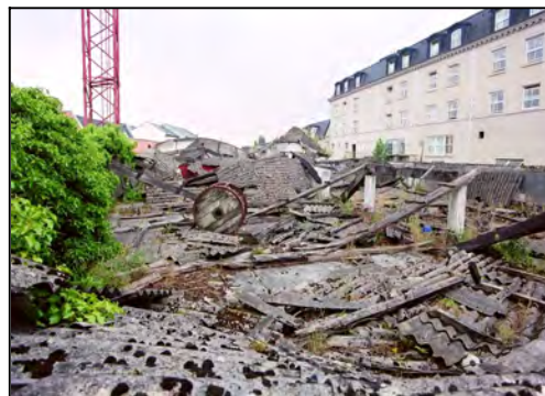
Fig 7.10 Going, going, gone ... Two views of different sections of the roof of a malt house at Tullamore (O17-064).
