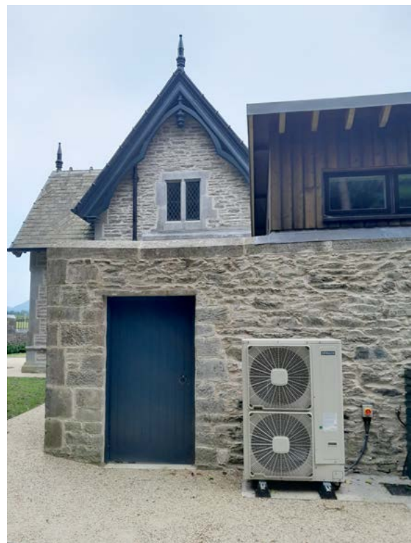
Figure 63: Air source heat pump
