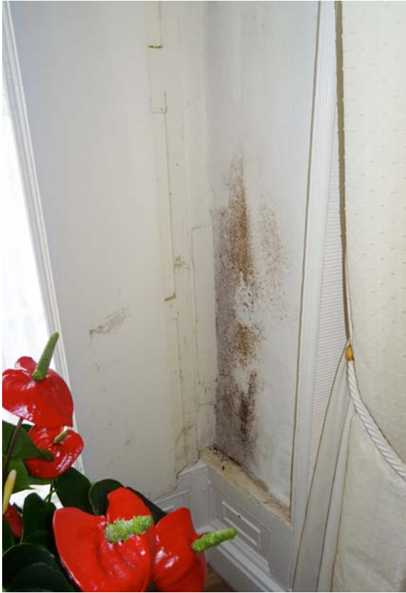
Figure 17: Mould growing behind shutters
