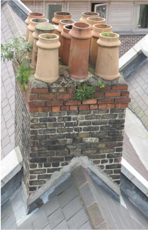
Figure 35: Traditional chimney stack requiring repair and maintenance
