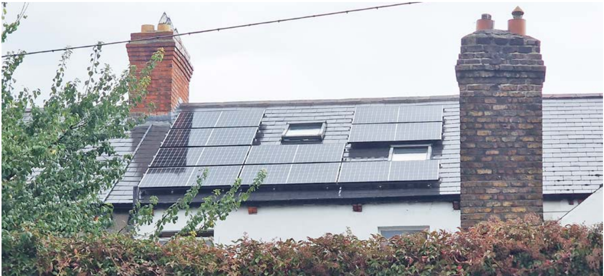
Figure 65: PV on the rear roof pitch of a traditional building
