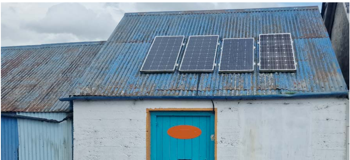
Figure 67: PV on the roof of an outbuilding
