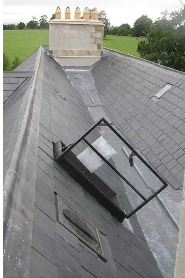
Figure 36: This modern double-glazed skylight allows access to a concealed valley gutter for maintenance inspections and cannot be seen from ground level (Image from Advice Series: Roofs , 2010)
