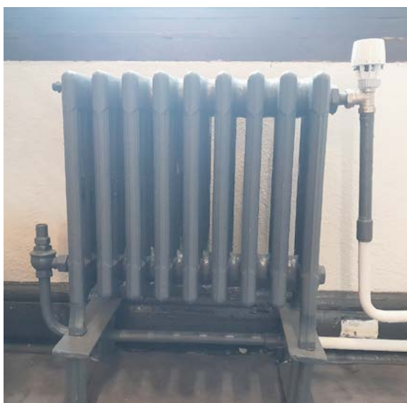
Figure 23: Cast-iron radiator with a thermostatic control
