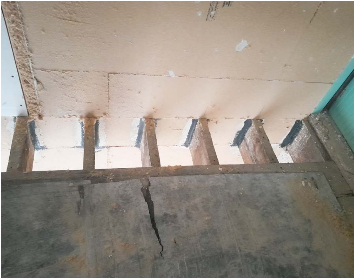
Figure 54: Woodfibre boards applied to walls and carefully fitted around and between floor joists to ensure continuity of insulation
