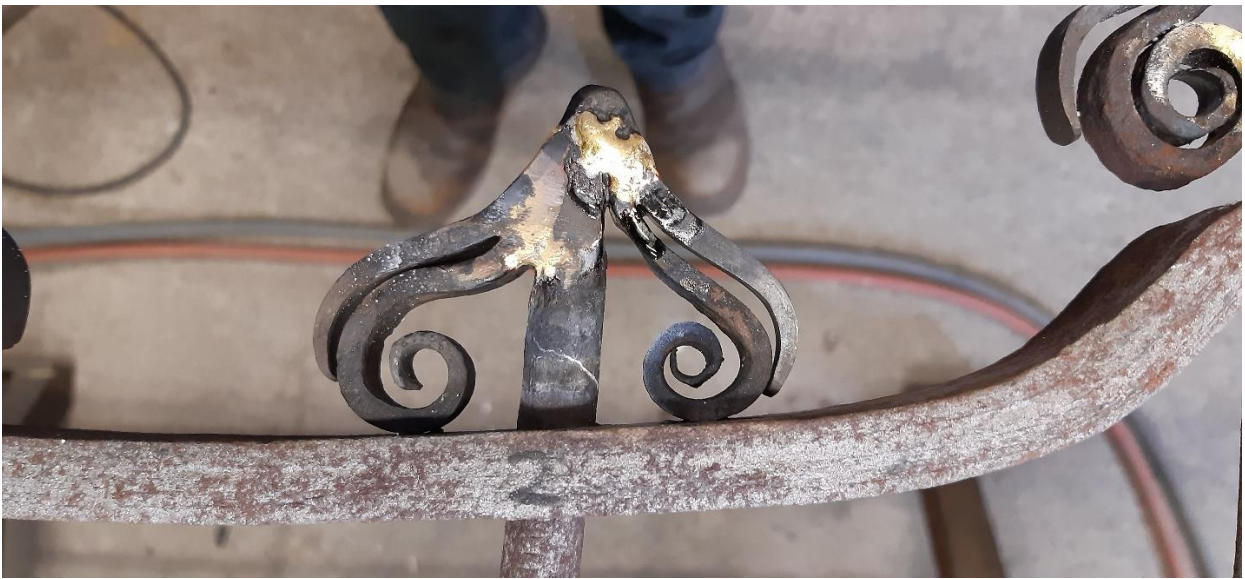
Stages in repairing a finial with new components which were first fire welded together then brazed onto the upright.
