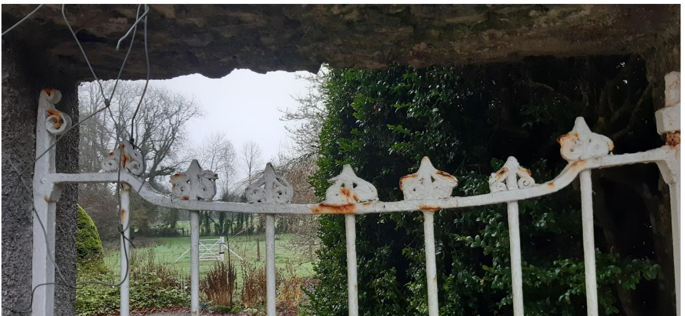
Poor condition of the top row of finials.
