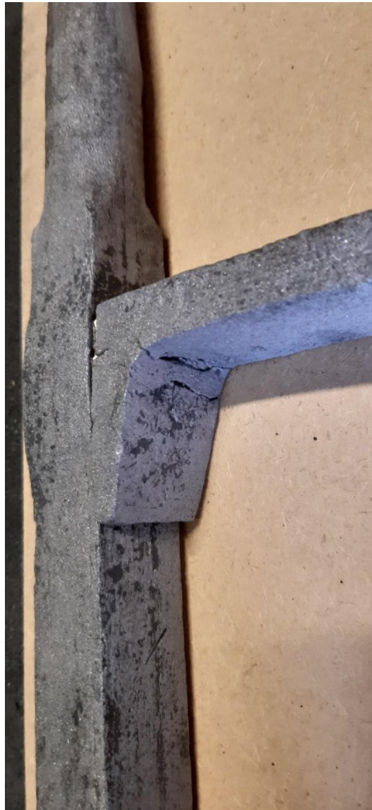
Fire welded gusset
