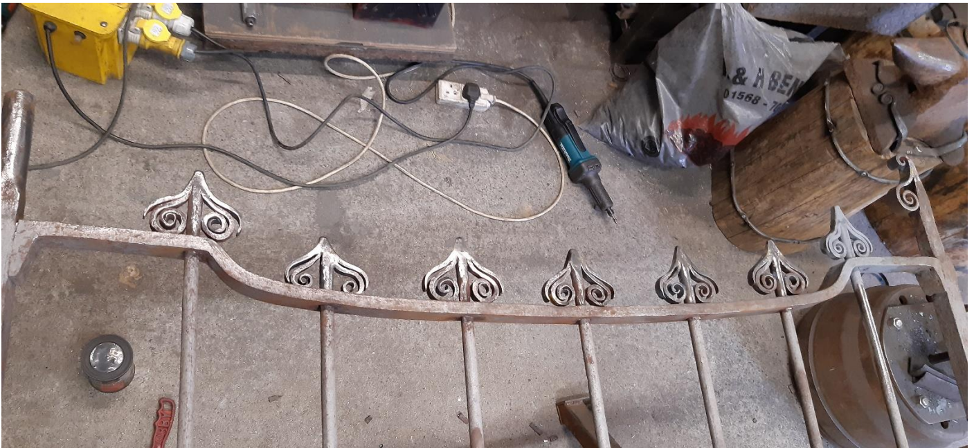
Before and after photographs showing all the repairs completed on the top row
