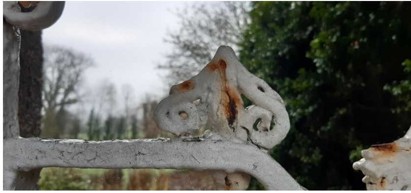
The corrosion can be clearly seen coming through the paint.
