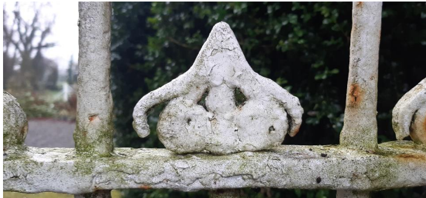
All the fine detail of the finials has been lost, hidden beneath the layers of corrosion and paint.
