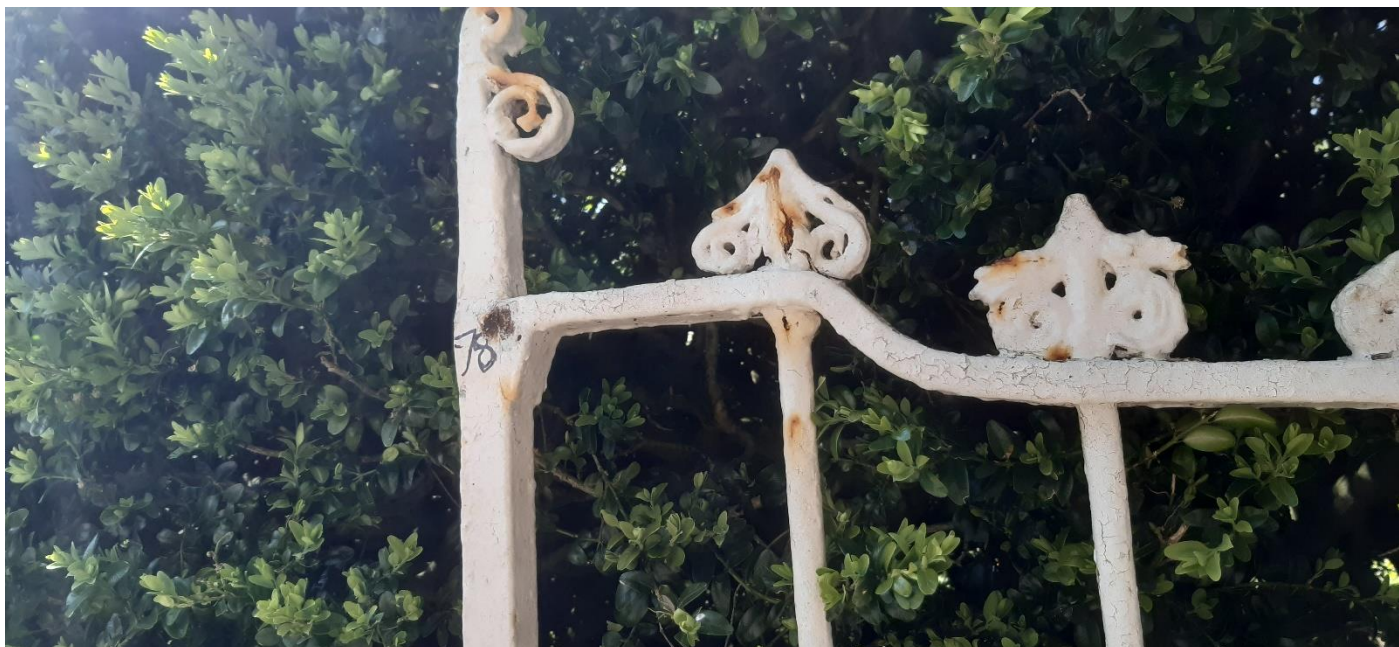
Close up showing the effect of “rust jacking”
