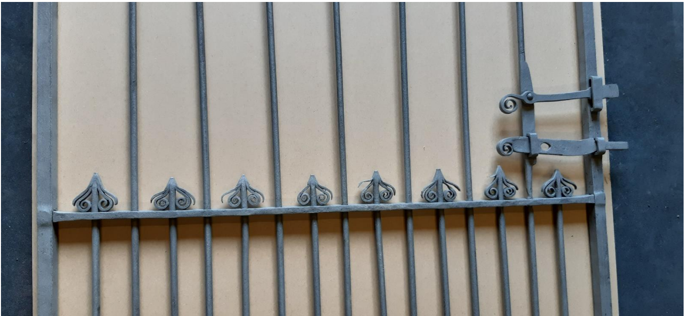
Before and after photographs showing all the repairs completed on the middle row
