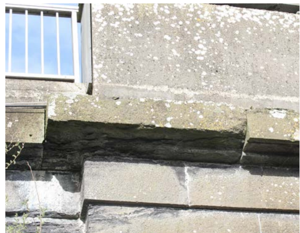
Fig. 99: Detail of damage to limestone cornice of Banagher Bridge
