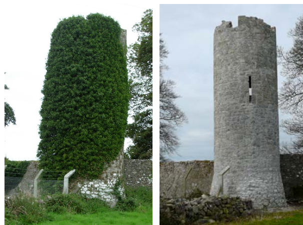
Fig. 150: Before and after image of the conservation and repair to a medieval tower at Athenry town wall by Howley Hayes Architects
