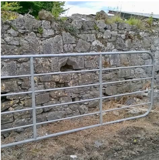
Fig. 23: Fifteenth-century ogee window lintel, recycled into the fabric of a rubble stone farmyard wall at Banagher. (Photo by E. Broderick)
