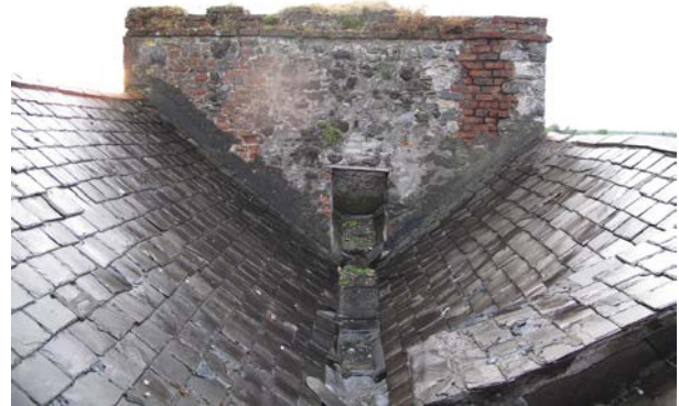
Fig. 64: Photograph of J.J. Hough's Singing Pub historic roof and chimney with doorway (Photo by E. Broderick)
