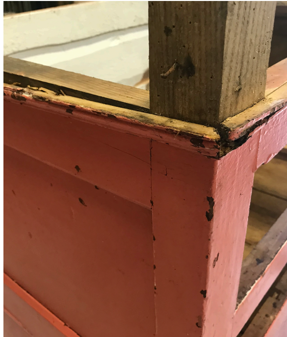
Damaged area to LH side miter
