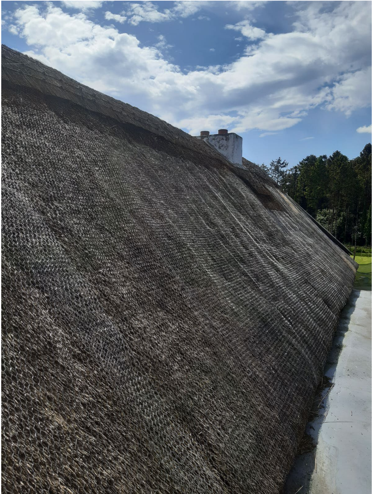
Chicken wire along length of roof, to prevent damage from high winds and birds. Decorative ridge repaired with hazel scallops.
