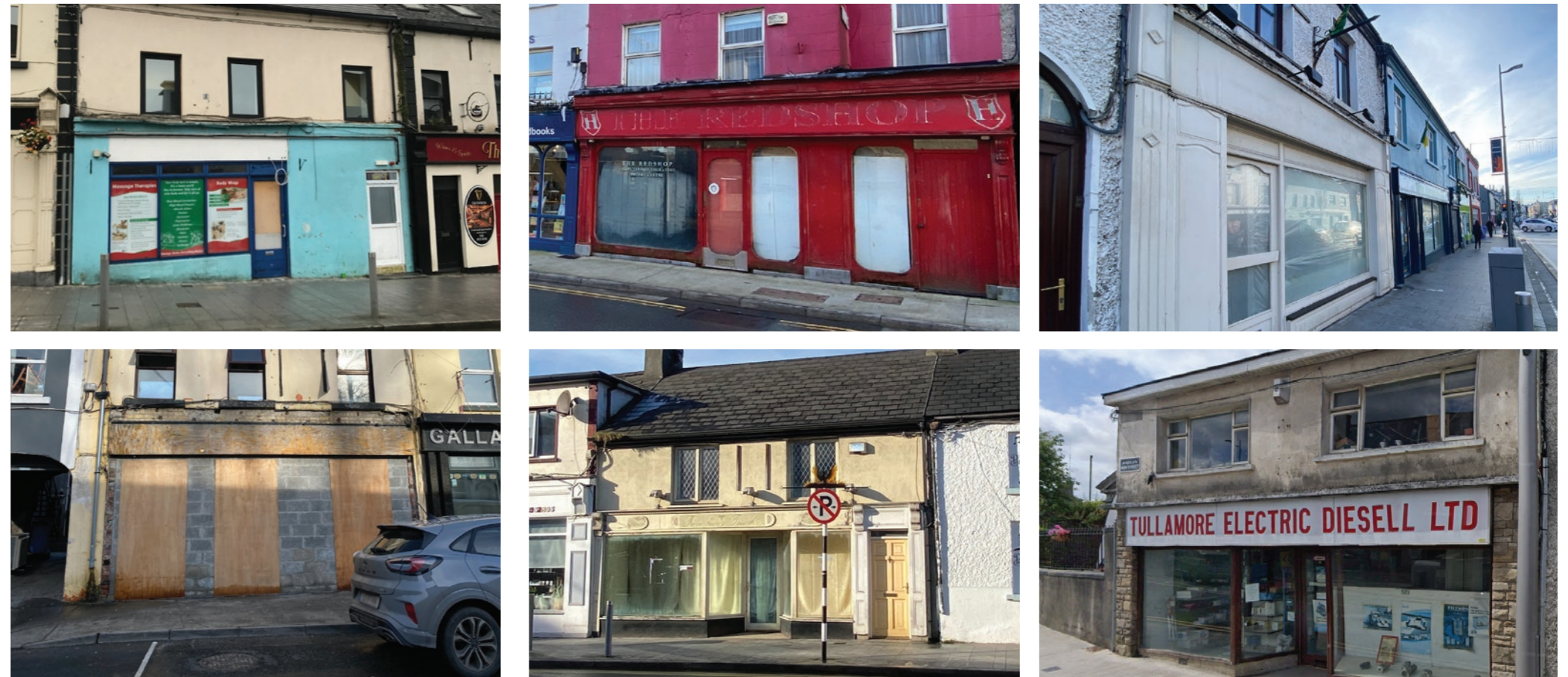
Examples of derelict and vacant shopfronts in Tullamore
