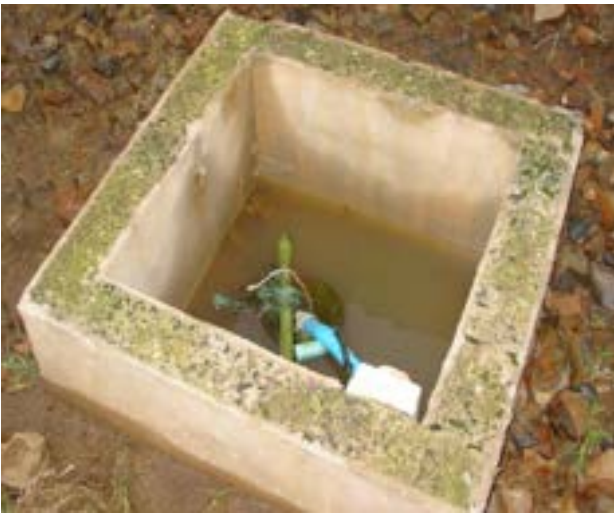
Figure 1: an unprotected borehole
