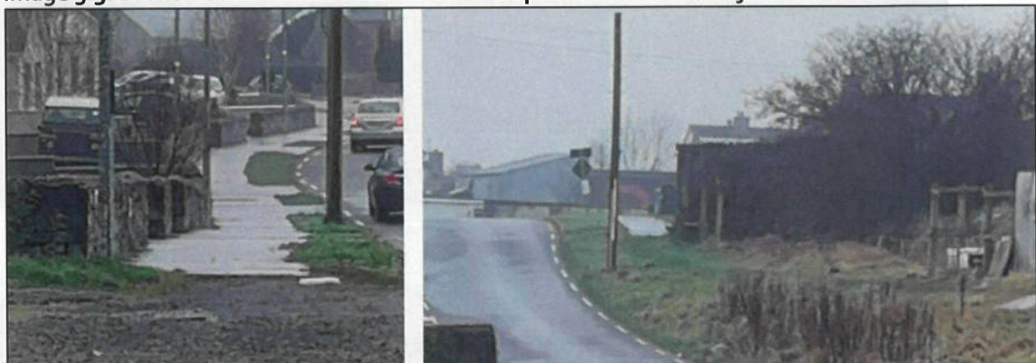
Image 3.3: Broken Connection between the Footpath due to the Subject Site
