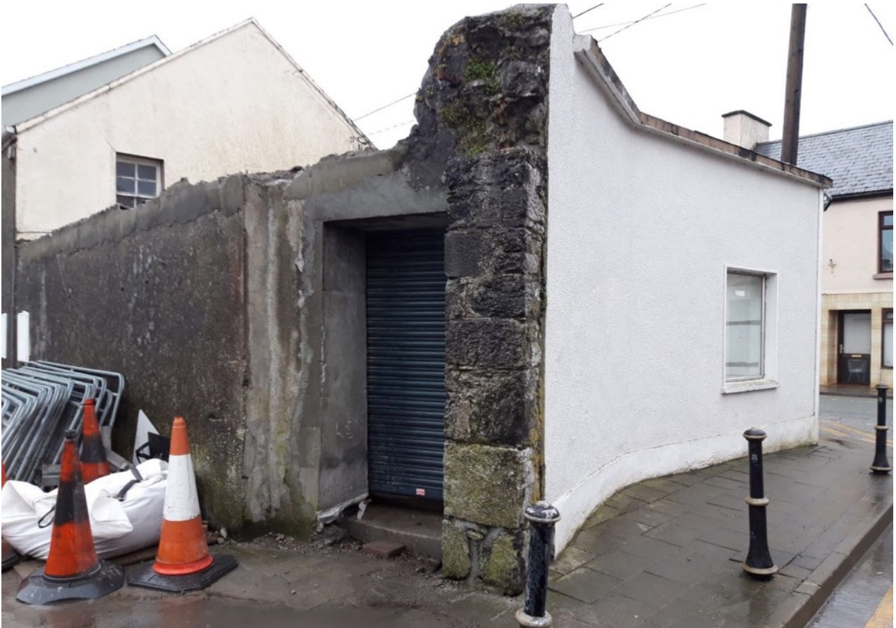
Plate 05: View from Crank Road of south gable with splayed detail in plan and evidence of former cut stone masonry arch and recent addition of door opening (February, 2020)
