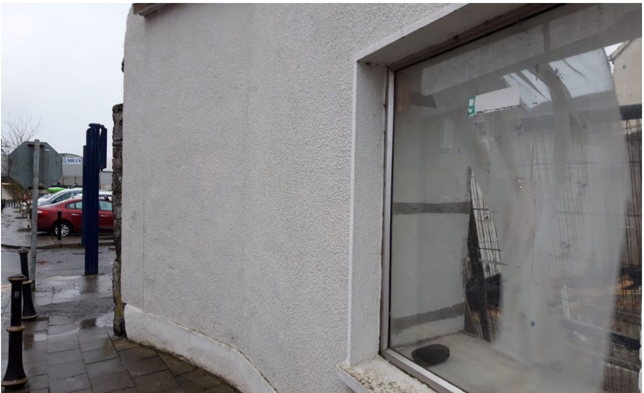
Plate 06: Detail of south gable facing onto Crank Road with splayed detail in plan and deep masonry construction as evidence by depth of internal window reveal (February, 2020)
