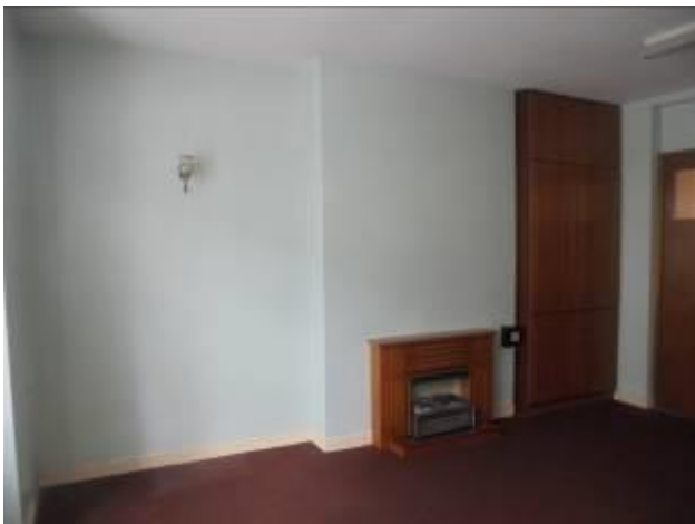
Figure 36: Fireplace at GF019
