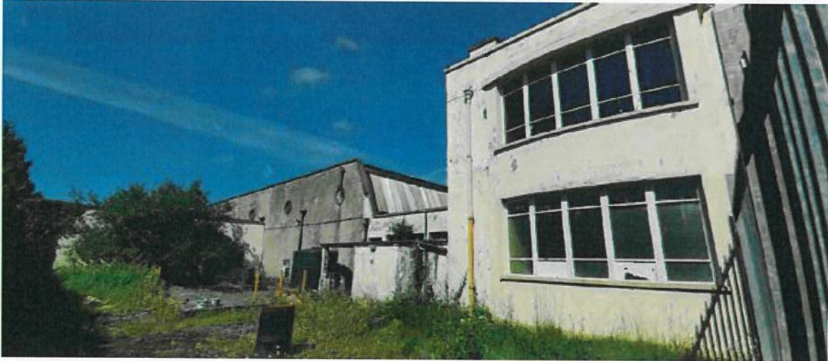
External view of flat roofed extension beside sawtooth building to rear of main building
