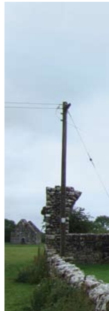
PLATE 26. Northwest view of nave and chancel church after removal of hard cement-rich coatings from the external walls.
