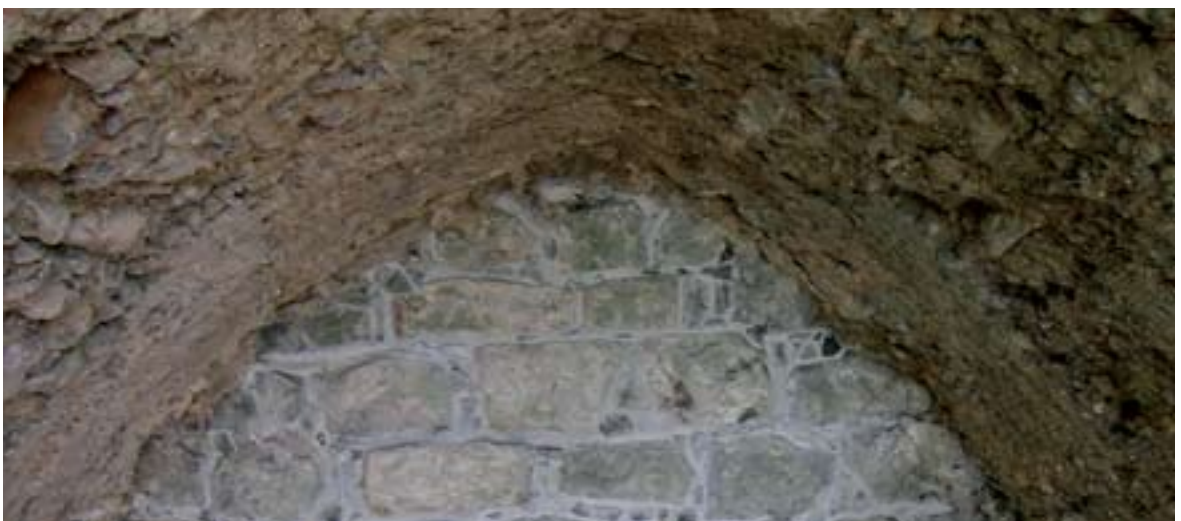
PLATE 57. View of barrel-vaulted chancel roof with traces of wicker-centring visible after removal of cement coating.
