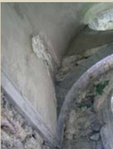
PLATE 17. Removal of hard cement-rich coatings from the underside of the stone-vaulted chancel.
