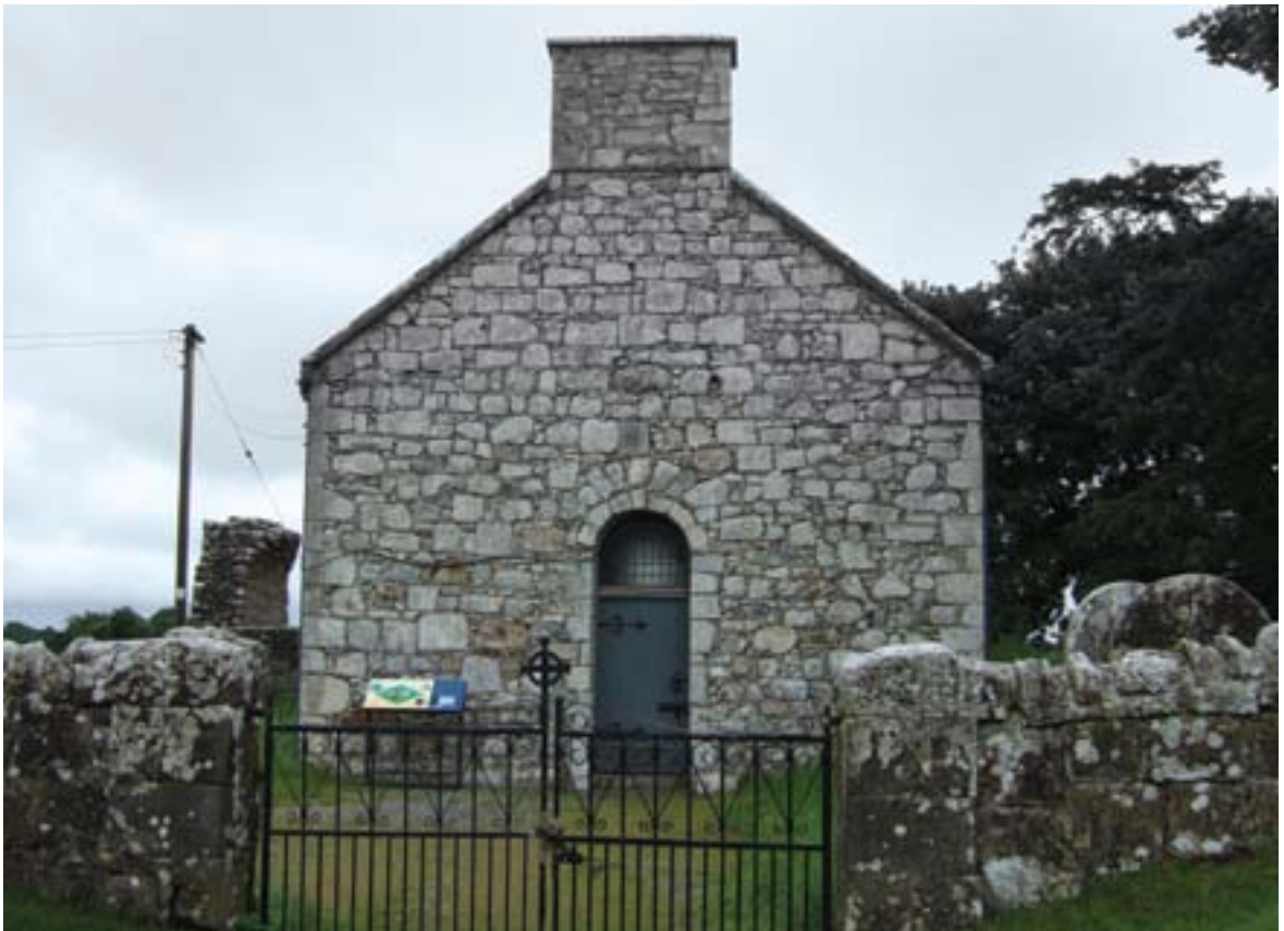
PLATE 55. External face of west gable showing historic fabric, main doorway and chimney stack rising from the apex of the gable.
