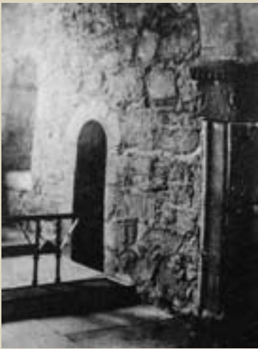
PLATE 15. View of internal face of the south wall of the chancel (Henry 1940).
