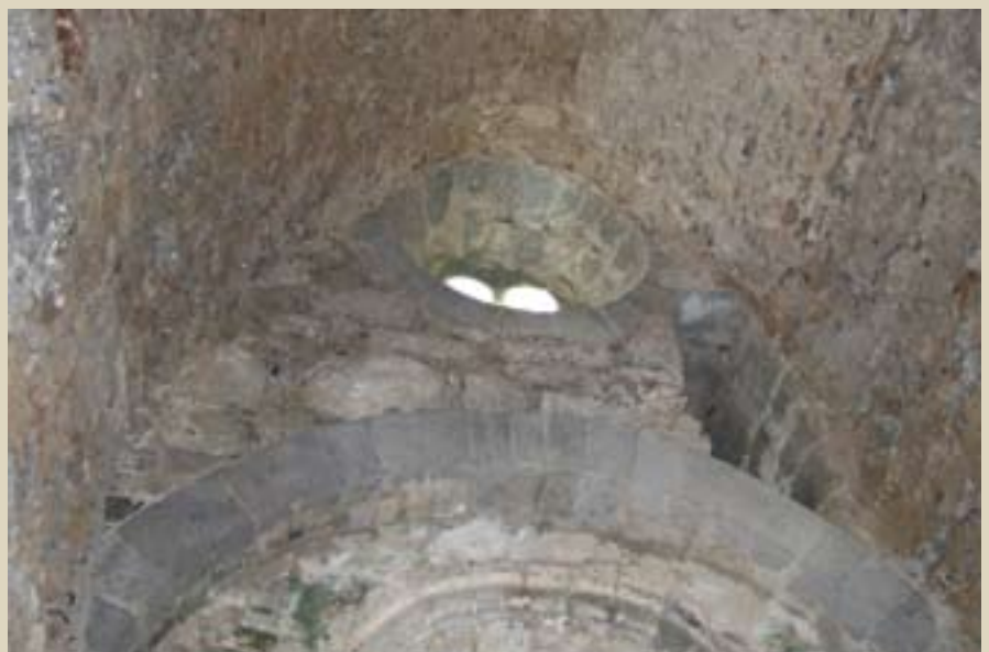
PLATE 19. View of the underside of the stone-vaulted chancel with evidence of wicker centring after removal of hard cement-rich coating.
