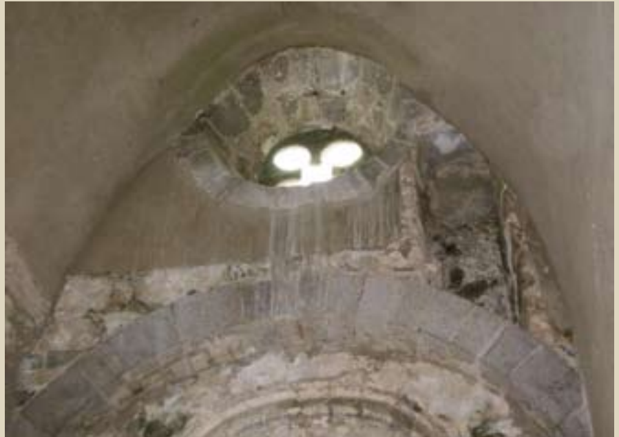
PLATE 18. View of the underside of the stone-vaulted chancel showing hard cement-rich coating prior to removal.
