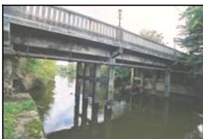
Fig 2.16a ( far left ): Lumcloon Bridge, on the Silver River, is a twin-span slab road bridge of 1949 (023-006).
