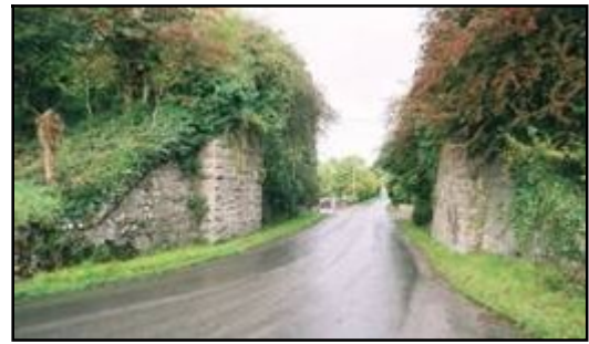
Fig 5.7 Only the abutments of this girder span survive on the Banagher line at Ballingowan Glebe (014-010).
