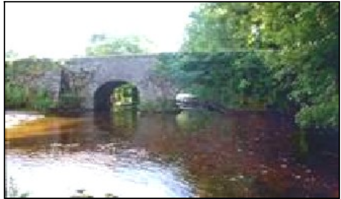
Fig 3.2 Ballynacarrig Bridge, over the Silver River has wide piers and narrow deck (032-001).
