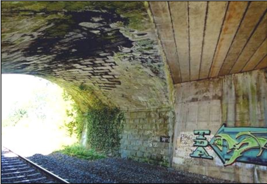
Fig 2.19 Concrete beam and slab extension to skew masonry arch road bridge over Dublin-Galway railway at Spol - lanstown (017-007).
