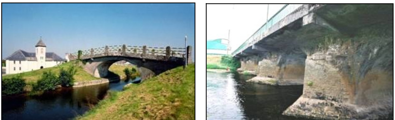
Fig 5.2a (left): Plunkett Bridge with its cantilevered footpaths and replacement railings (015-015). Fig 5.2b (right): Cantilevered concrete footpath, Barrow Bridge (034-005)
