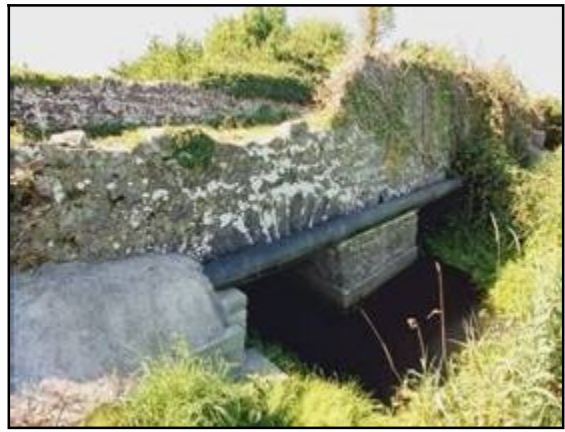
Fig 5.8 Damaged parapet at Derrygolan Bridge (009-007).
