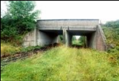
Fig 2.17a ( far left ): Replacement concrete slab deck on masonry abutments of rail/road bridge, Srah Td (017-098);
