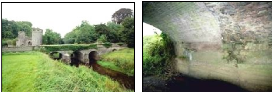
Fig 2.10 Mucklagh Bridge (016-029), over the Clodiagh River at Charleville, was widened on its upstream side with mass concrete arches.
