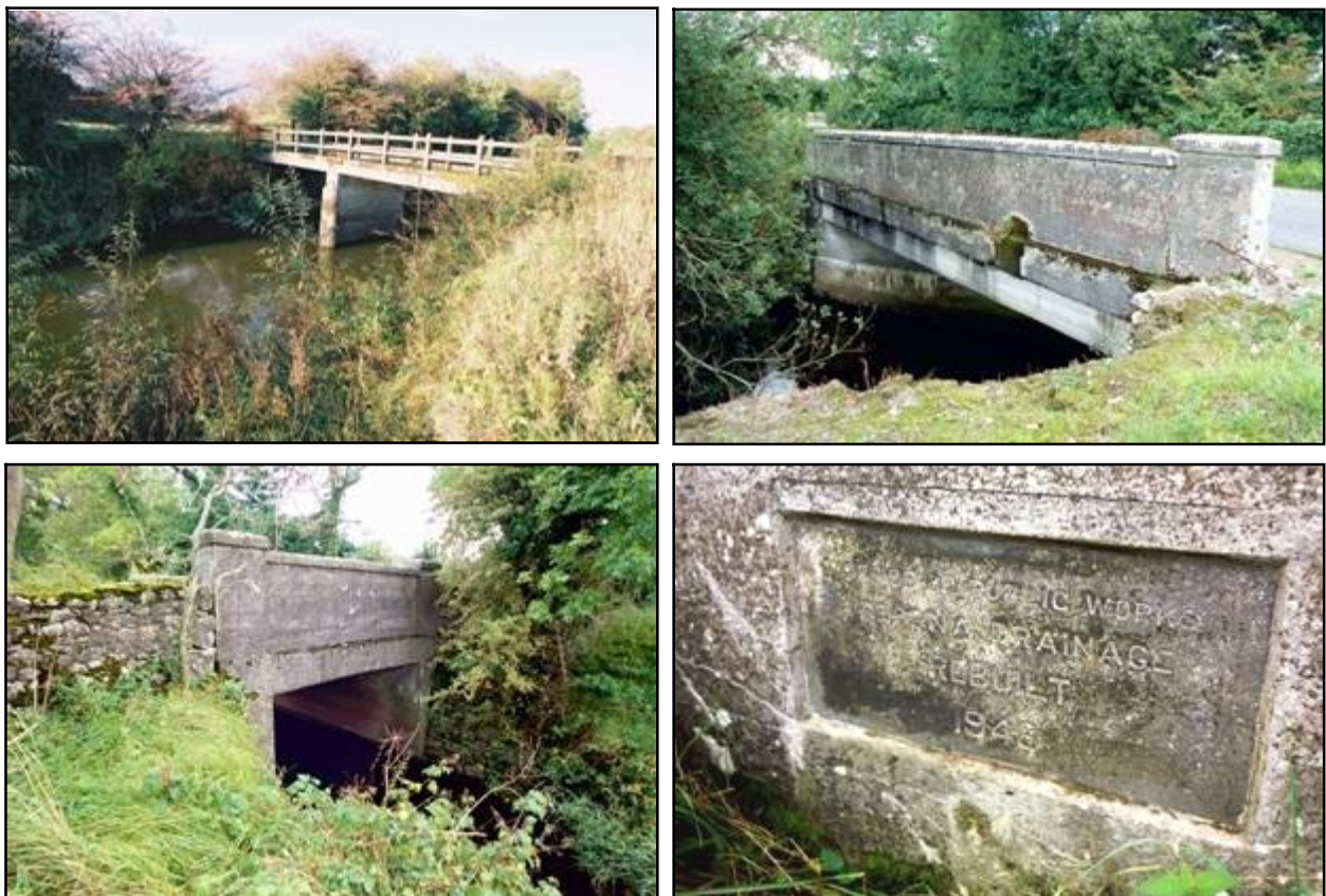
Fig 3.30a (top left): Accommodation bridge over River Brosna, Ballycumber (007-024). Fig 3.30b (top right): Barnaboy Bridge over Silver River, Kilnagall Td (031-002). Fig 3.30c (bottom left) Road bridge over tributary of Brosna, Clonony Beg Td (022-030). Fig 3.30d (bottom right): 1948 datestone on Clonony Beg bridge.
