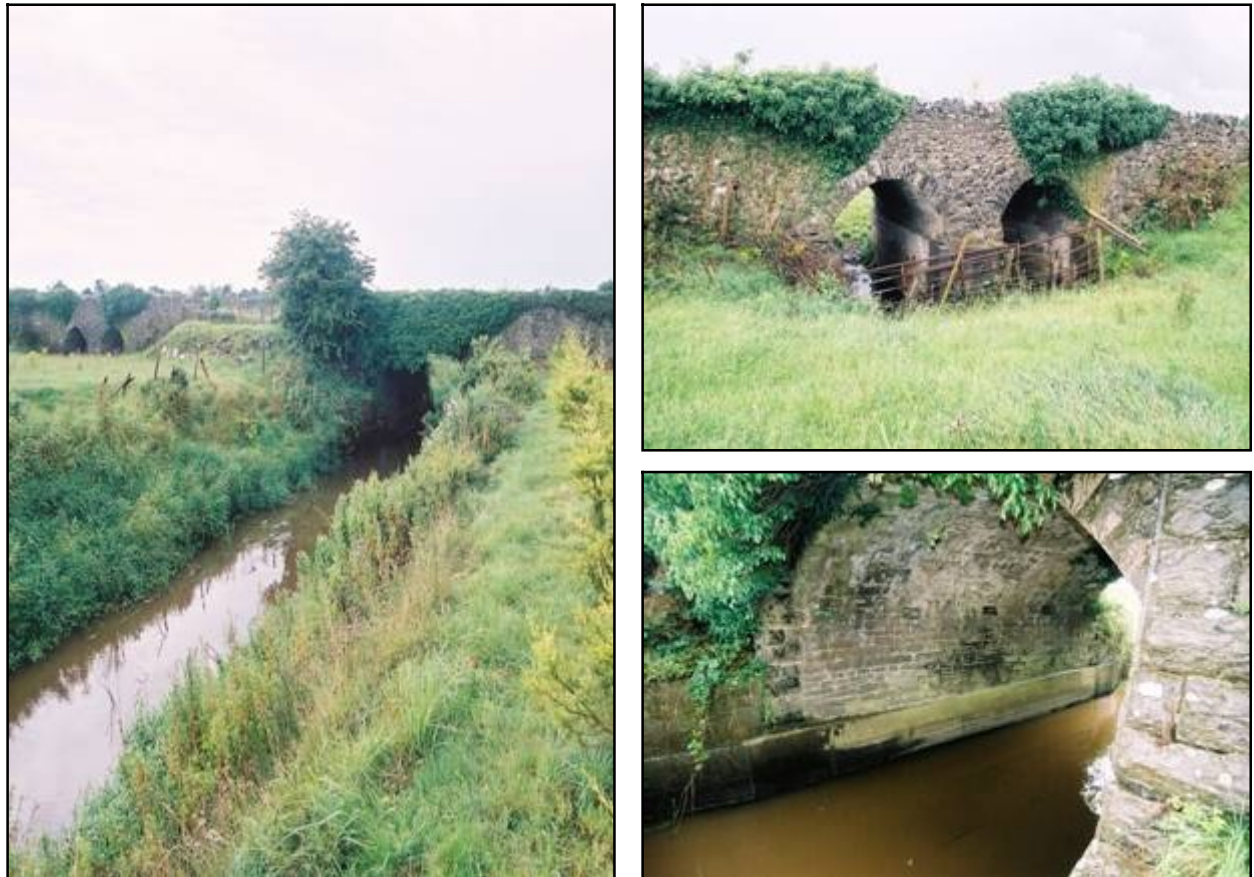
Fig 3.16 At Baltinoran Bridge (004-001), the Mongagh River was straightened ( left ) and the former rubble stone causeway bridge ( top right ) extended with a new dressed stone bridge ( bottom right ).
