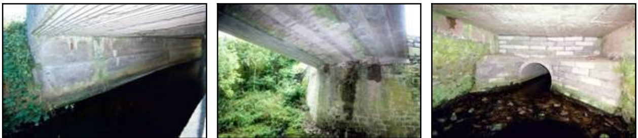
Fig 5.1a (left): Corrugated metal sheeting was used as falsework for this concrete slab extension to Gormagh Bridge over the Silver River (009-004). Fig 5.1b (middle): Pre-cast concrete beams were added along both sides of the existing concrete slab deck of this road bridge over the former Shannon Navigation at Clonahenoge Td (029-003). Fig 5.1c (right): The slab deck of Little Bridge, Kilmaine Td, was widened with a concrete pipe (036-003).
