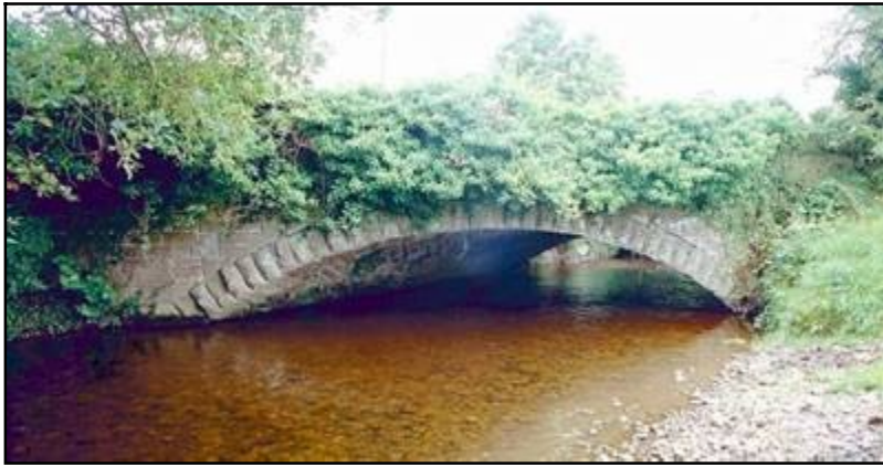
Fig 4.3 Carrig Bridge (036-006), a shallow skew span Board of Works construction of 1852 over the Camcor River.
