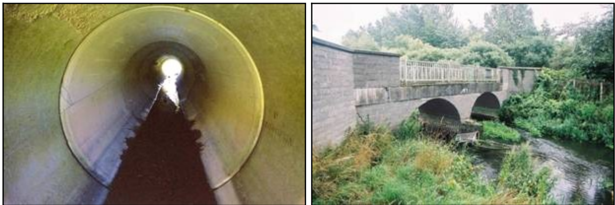
Fig 2.22a ( left ): This concrete pipe carries a drain under a road in Cloncollog Td (017-043). Fig 2.22b ( right ): Twin-span Armco footbridge of c.1970 over the Tullamore River, O'Molloy St, Tullamore (017-094).
