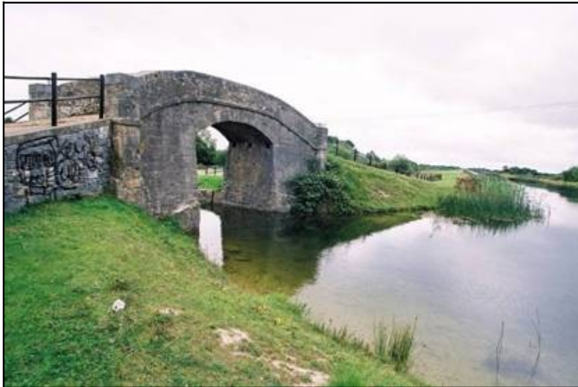
Fig 3.10 Downshire Bridge (012-013). The main line of the Grand Canal is on the right, with the Edenderry branch passing under the bridge at left.
