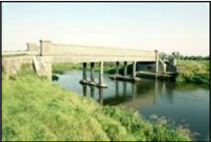
Fig 2.1a (left): Belmont Bridge, an 18 th century five-arch masonry road bridge over the River Brosna (014-005).
