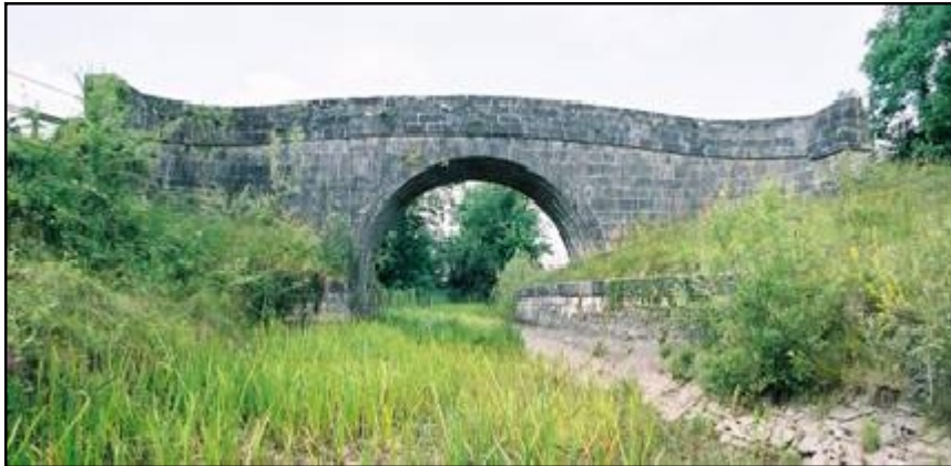
Fig 3.12 Tony's bridge carries an accommodation track over the Kilbeggan Canal, Wood of O Td (017-029).
