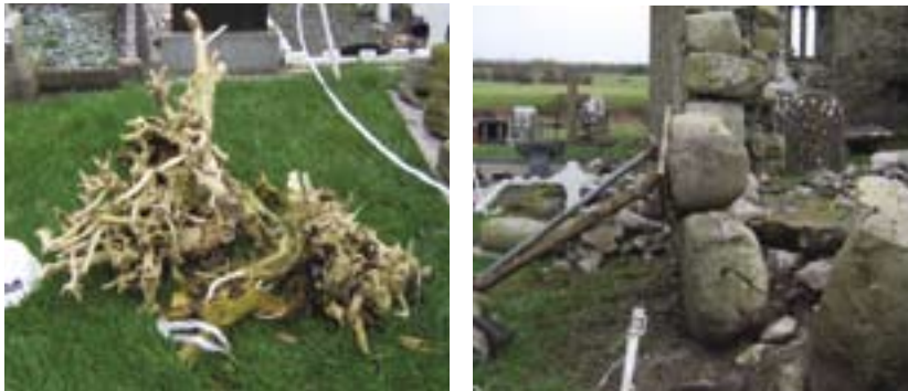
Ivy root system removed from Northwest corner NW corner following removal of ivy
