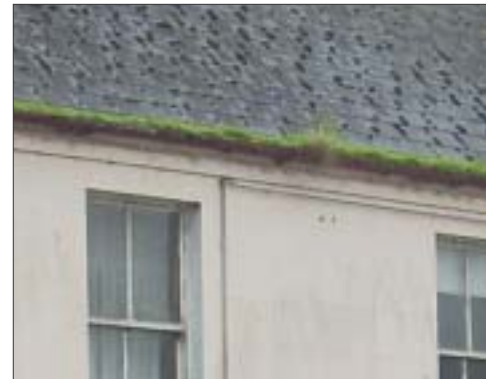
Market Square: Vegetation invading gutters
