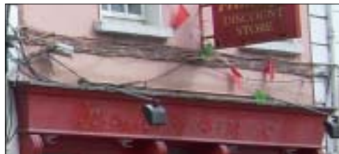
Main Street: Signage needing maintenance
