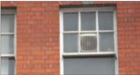
Emmet Square: Window fan unit undermines visual integrity
