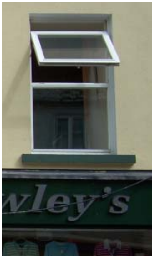
Main Street: Inappropriate window type
