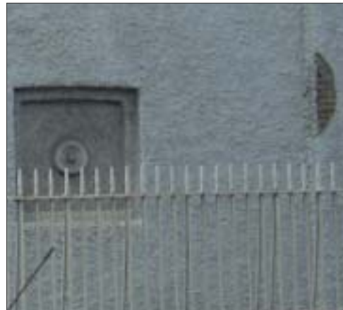
Courthouse: Wall finish chipping away on the facade
