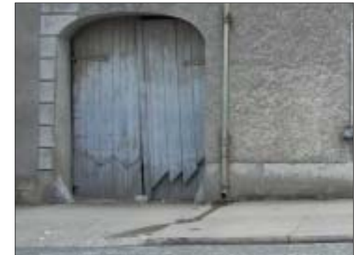
Townsend Street: Gate needing repair
