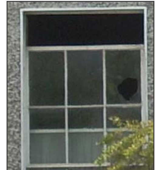
John's Place: Broken window on Georgian facade
