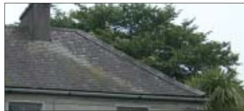
Townsend Street: Home needing roof maintenance
