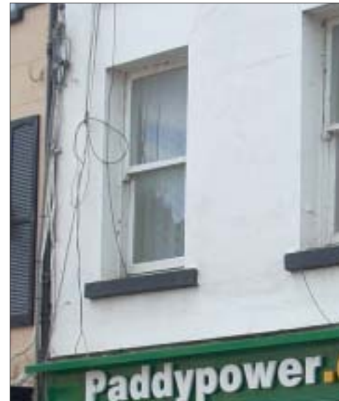
Main Street: Cabling causing visual clutter
