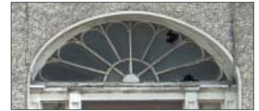
Emmet Street: Broken window on Georgian facade
