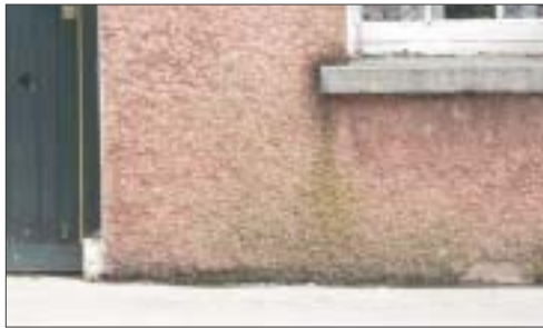
Rosse Row: Mold/mildew stains on window sill and wall
