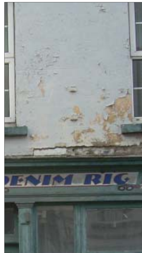
Connaught Street: Painting peeling off facade
