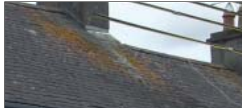
Rosse Row: Homes needing roof maintenance
