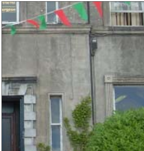
Emmet Square: Stained masonry facade
