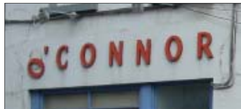
Main Street: Signage needing maintenance
