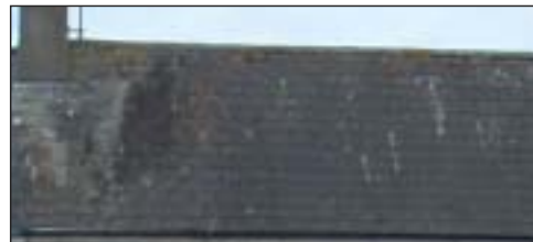
Emmet Square: building needing roof maintenance
