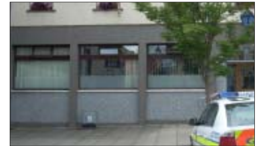
Emmet Square: Stone cladding inappropriate
