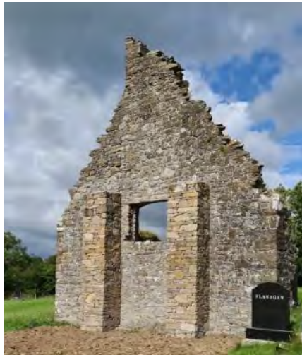
Roscomroe medieval church gable end after stabilisation works carried out with National Monuments Service consents.
