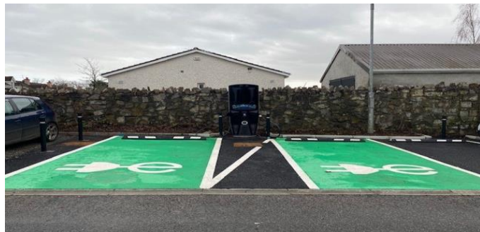
Electrical Vehicle Charging Point at Aras an Chontae
