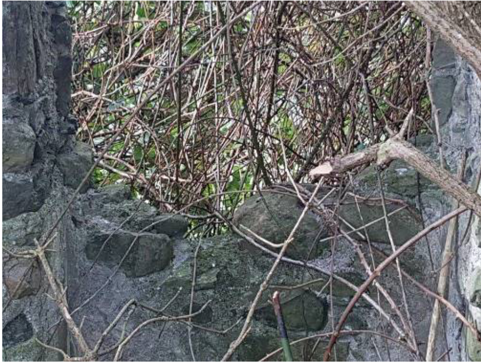
10. Some cills require minor rebuilding.
