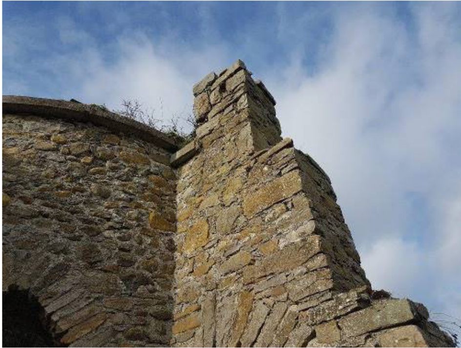
14. One buttress shows stonework above eaves and indicates that all buttresses would be at least as high.
