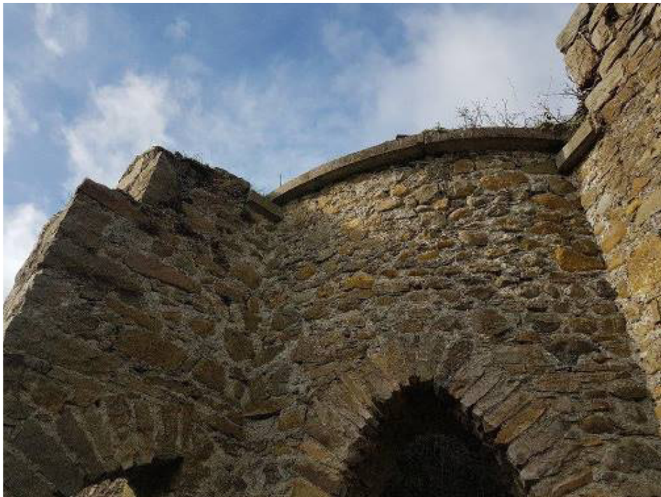
13. Sloping stonework appears to be missing from flying buttresses and requires restoration.
