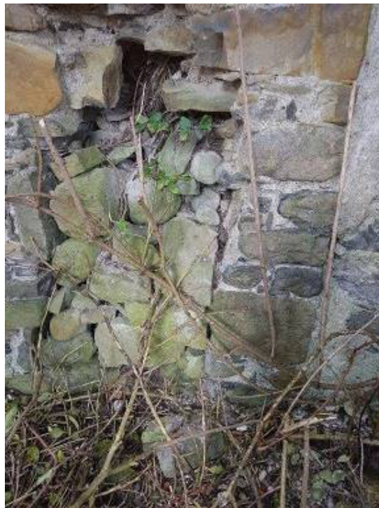
9. Blocked up fireplace to be unblocked.
