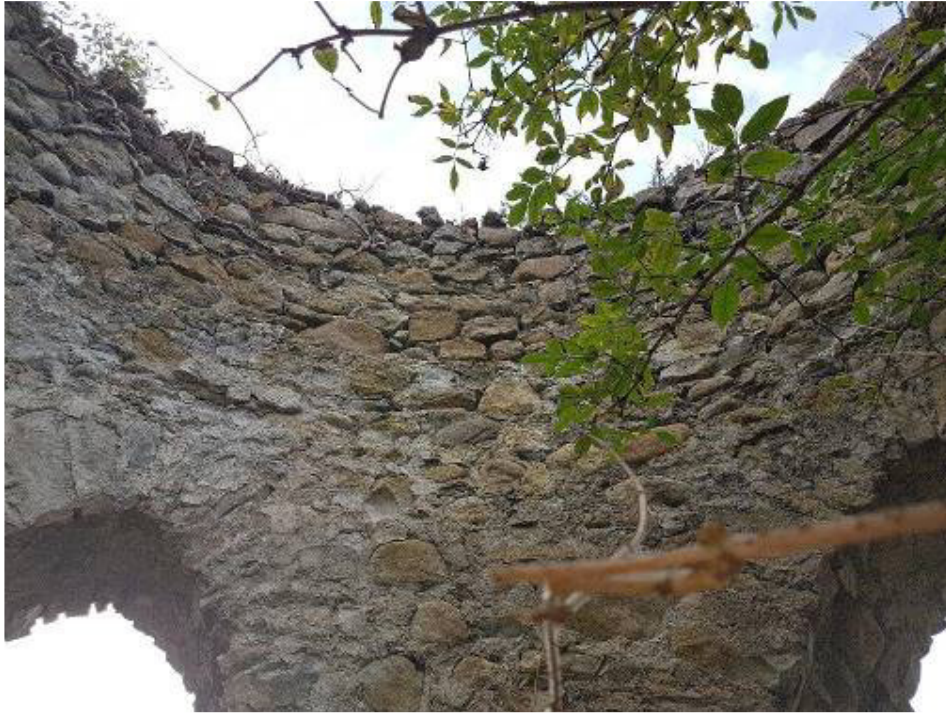
12. Some consolidation to top 1m of stonework is required.
