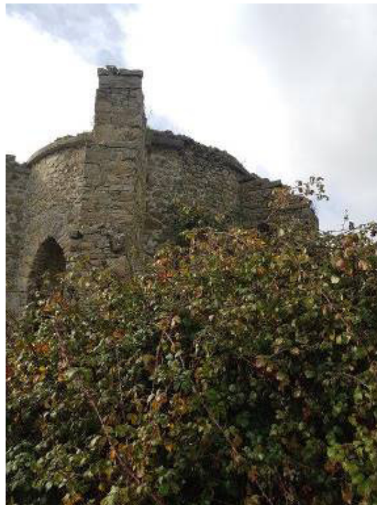
14.1 View of highest buttress. Giving evidence that all buttresses were once well above eaves level
