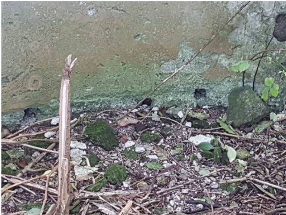
17. Spalled masonry from the top of the walls
