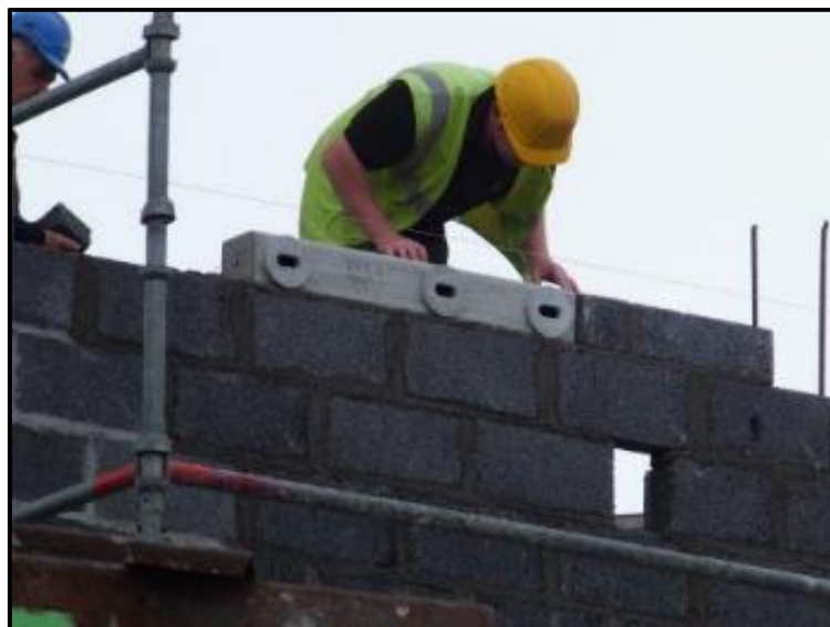
Figure 32. Installing Swift boxes as part of the fabric of the wall. Photo: Lynda Huxley (Swift Conservation Ireland).
