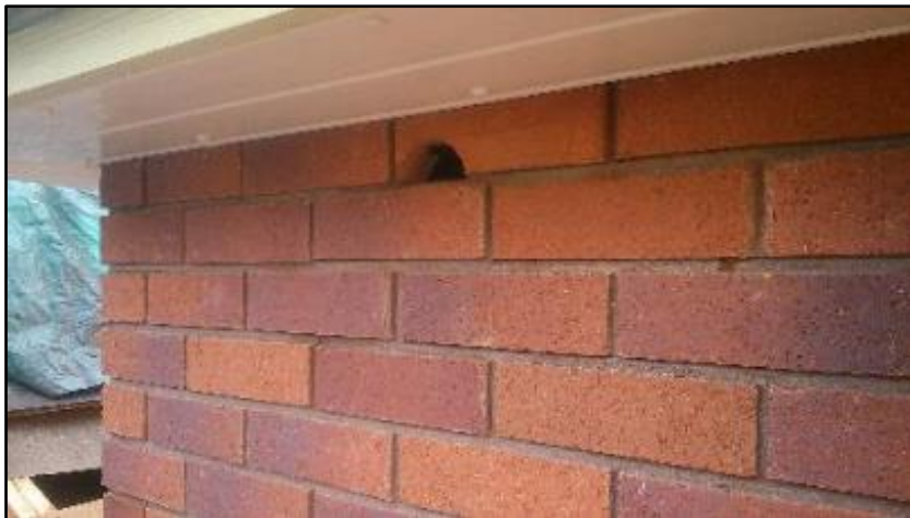
Figure 34. A Swift Brick installed in a newly erected redbrick wall. Photo: www.birdbrickhouses.co.uk .
