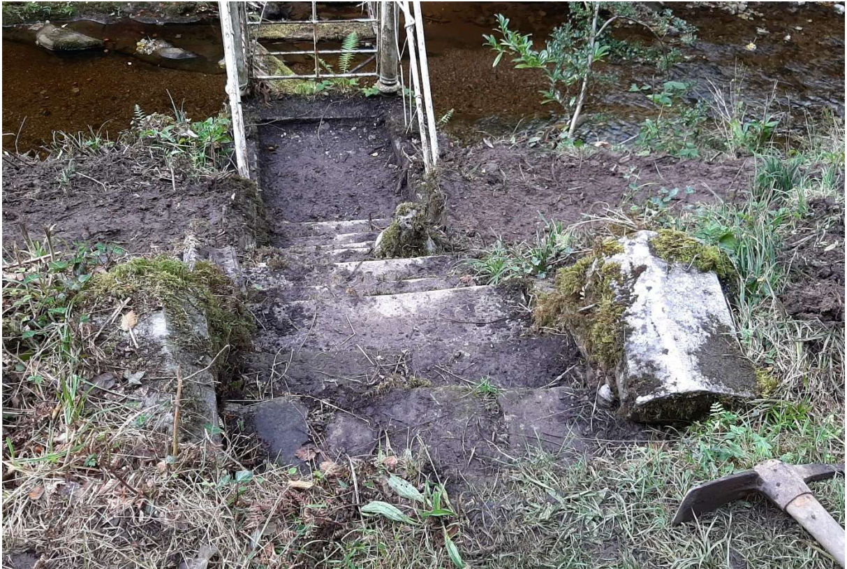
Stone steps and cappings uncovered as part of clearing and site preparation
