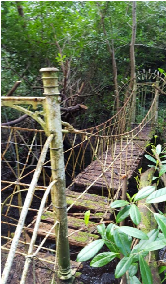
Prior to works, missing sections
