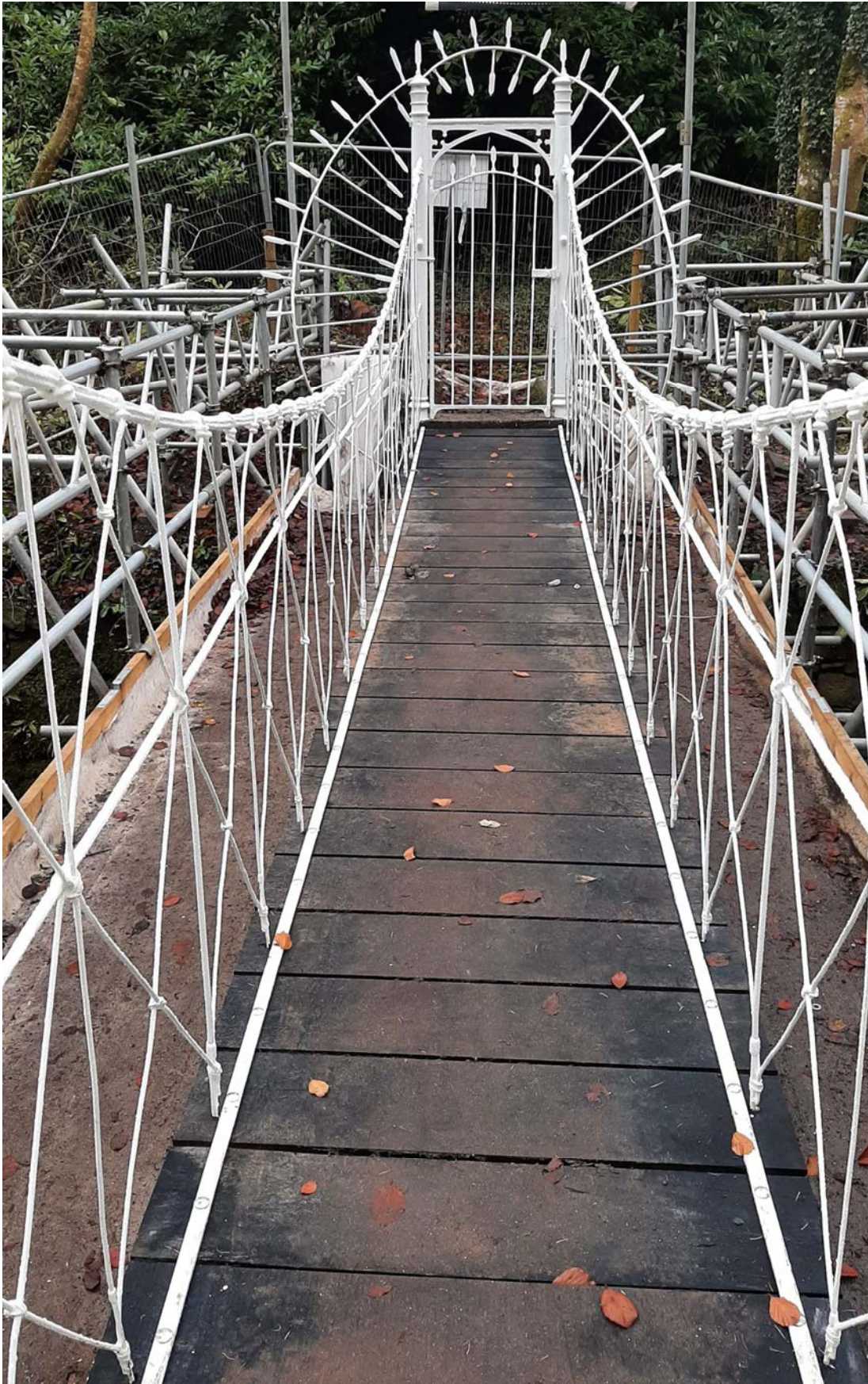
New timber deck with Oak from the estate by Coillte, diagonal supports and the delicate connection through new decking to horizontal bar below as per original detailing
