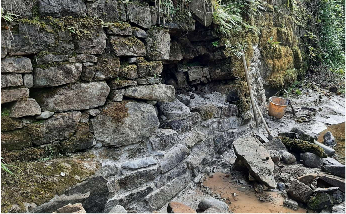
Sections of embankment washed out requiring repair with lime mortar
