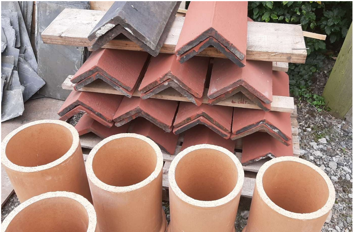
2021_0708 Slating continues, repairs to gable. Flues for chimney and terracotta ridge tiles
