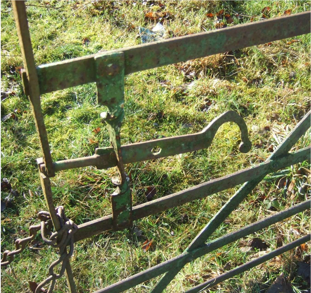
Prior to repair
