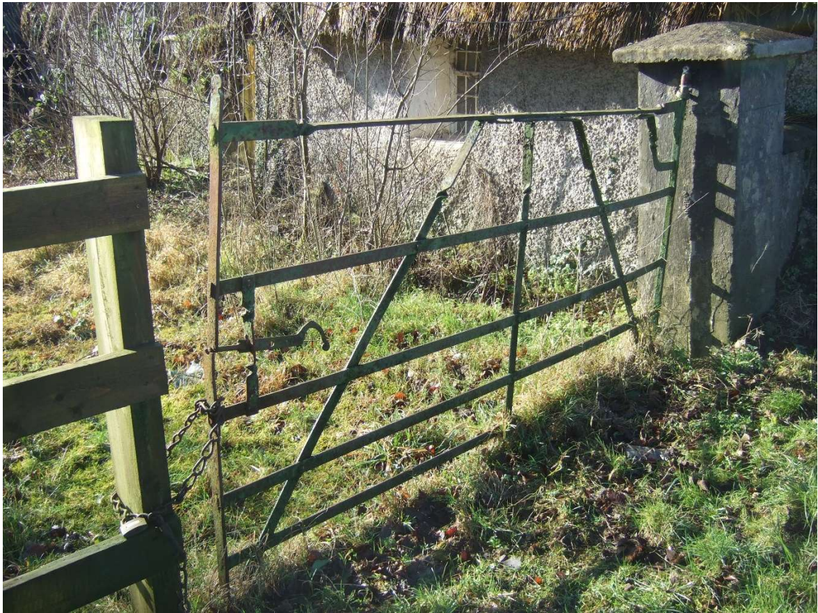
2016_0216 Wrought Iron gate on site – sections bent or broken
