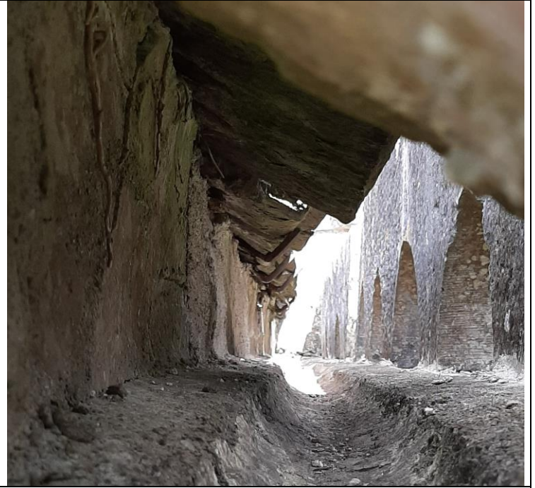
14. Ditto. While the flag roof over sails the valleys in areas the camber of the surface on either side of the valley, now cleared, should allow overshooting water to run back down into the valley and away
