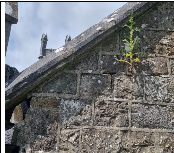
7. End coping stones to be rebuilt in phase 2
