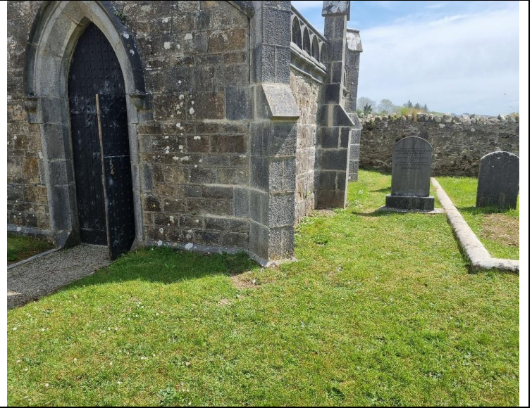
2. Typical buttress which has had helibars ties and stainless-steel threaded rod tying at kneeler position
