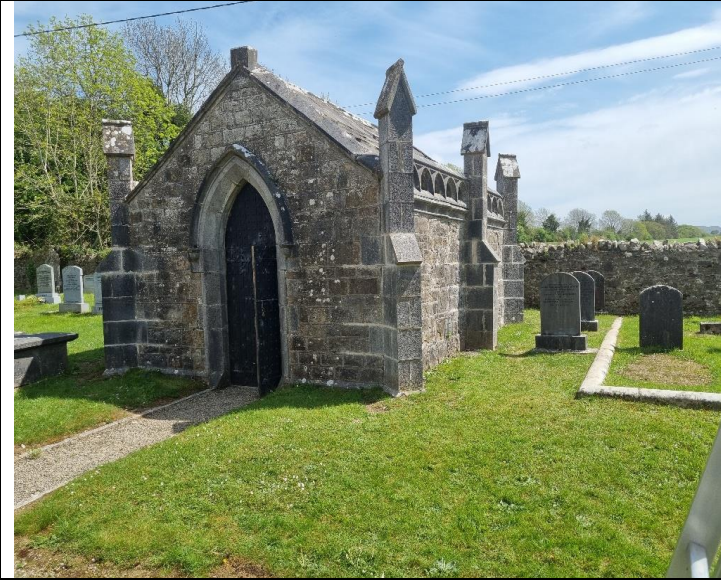
1. The completed project for phase 1 which has had the temporary ties removed.
