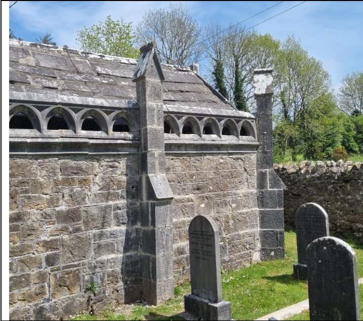
5. All cast iron cramps will need to be removed and the stonework numbered and rebuilt in phase 2
