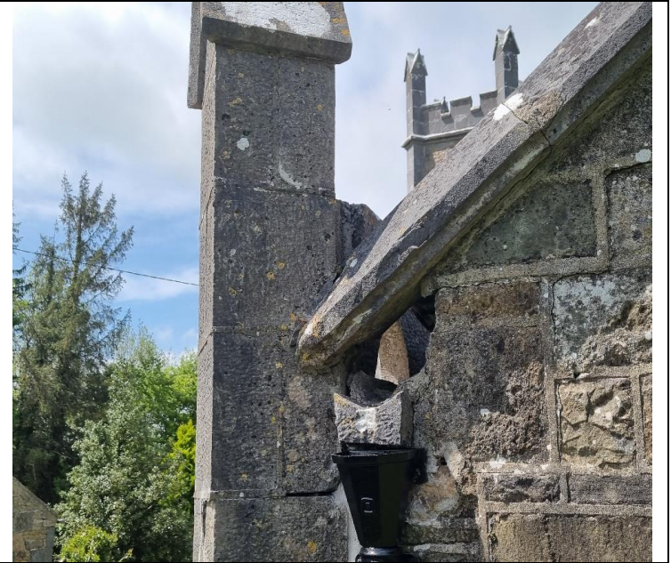
6. The upper level of the SE buttress has also displaced from Iron cramp corrosion and will need rebuilding in phase 2
