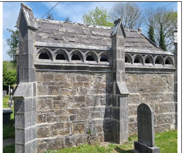
4. The high level tracery has been fixed historically with wrought iron cramps which have corroded causing opening of cracks
