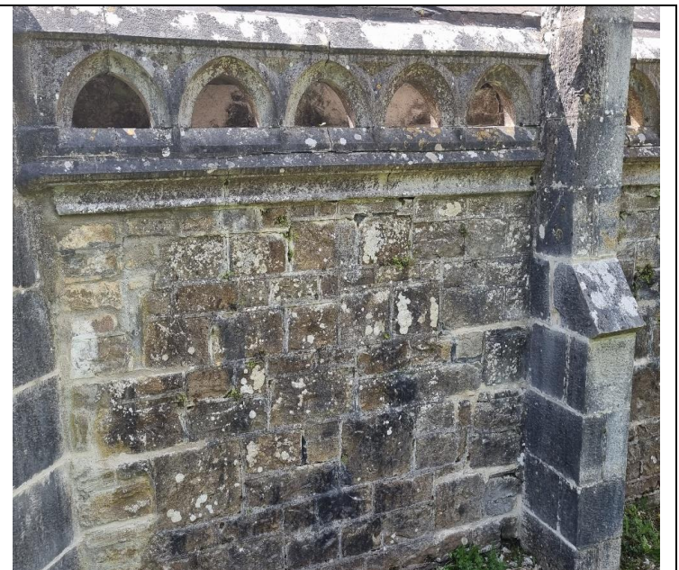
8. Note the top course of rubble masonry has moved due to iron cramp expansion to be addressed in phase 2
