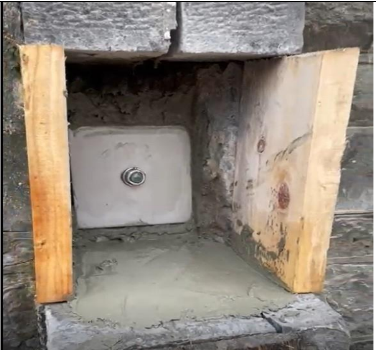
12. Stainless steel tie rod and plates during installation. These stabilise and tie the tall and narrow decorative buttresses to the main structure.
