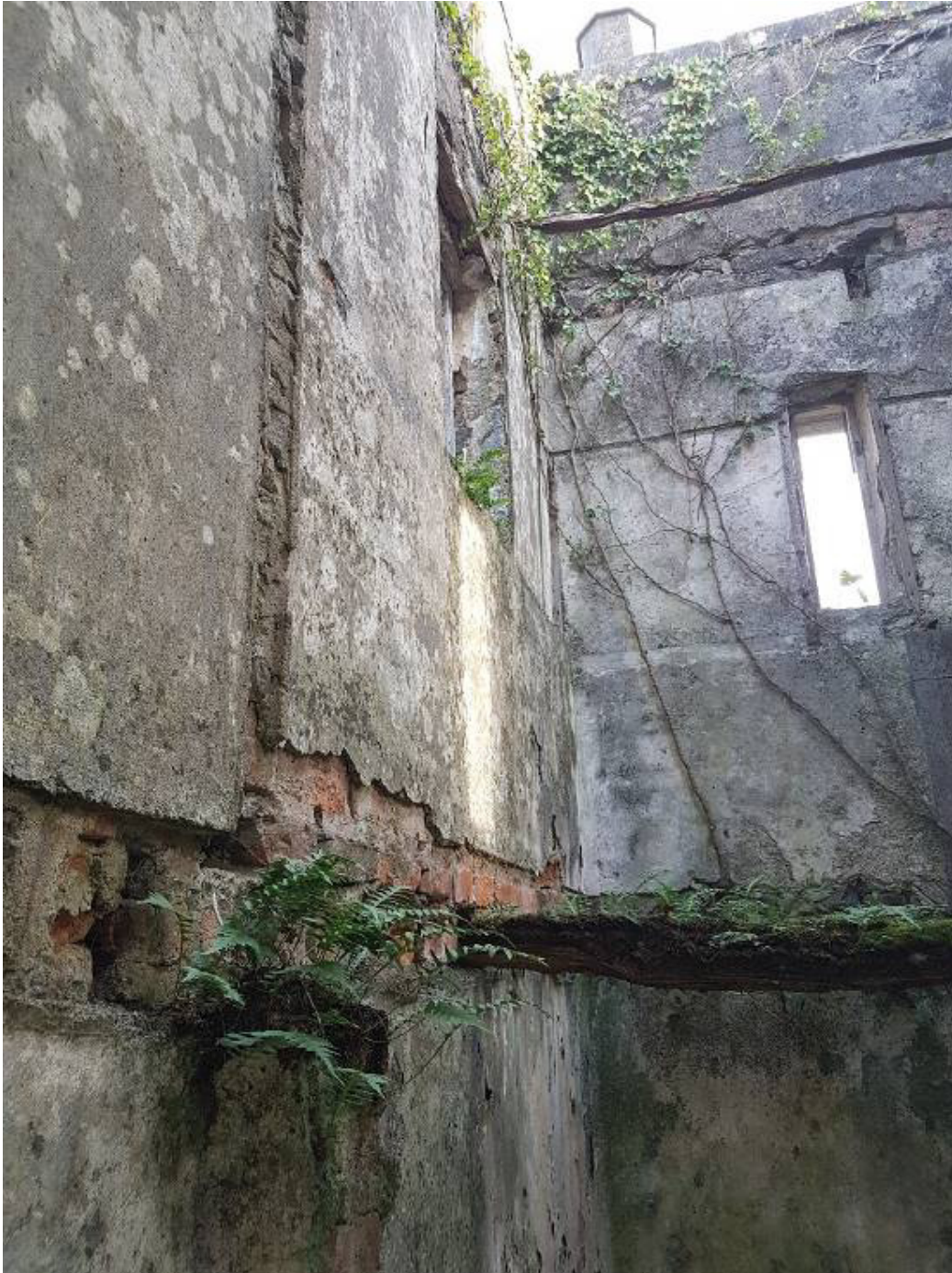
General view of first floor level. Ivy and vegetation -minor treatment. Timber joists to be removed lintels to be replaced in precast concrete. Plaster to remain unless unstable.
