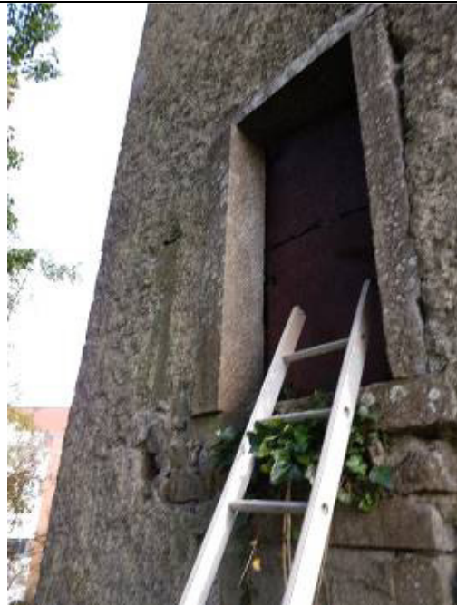
South West ladder access where external stairs is missing
