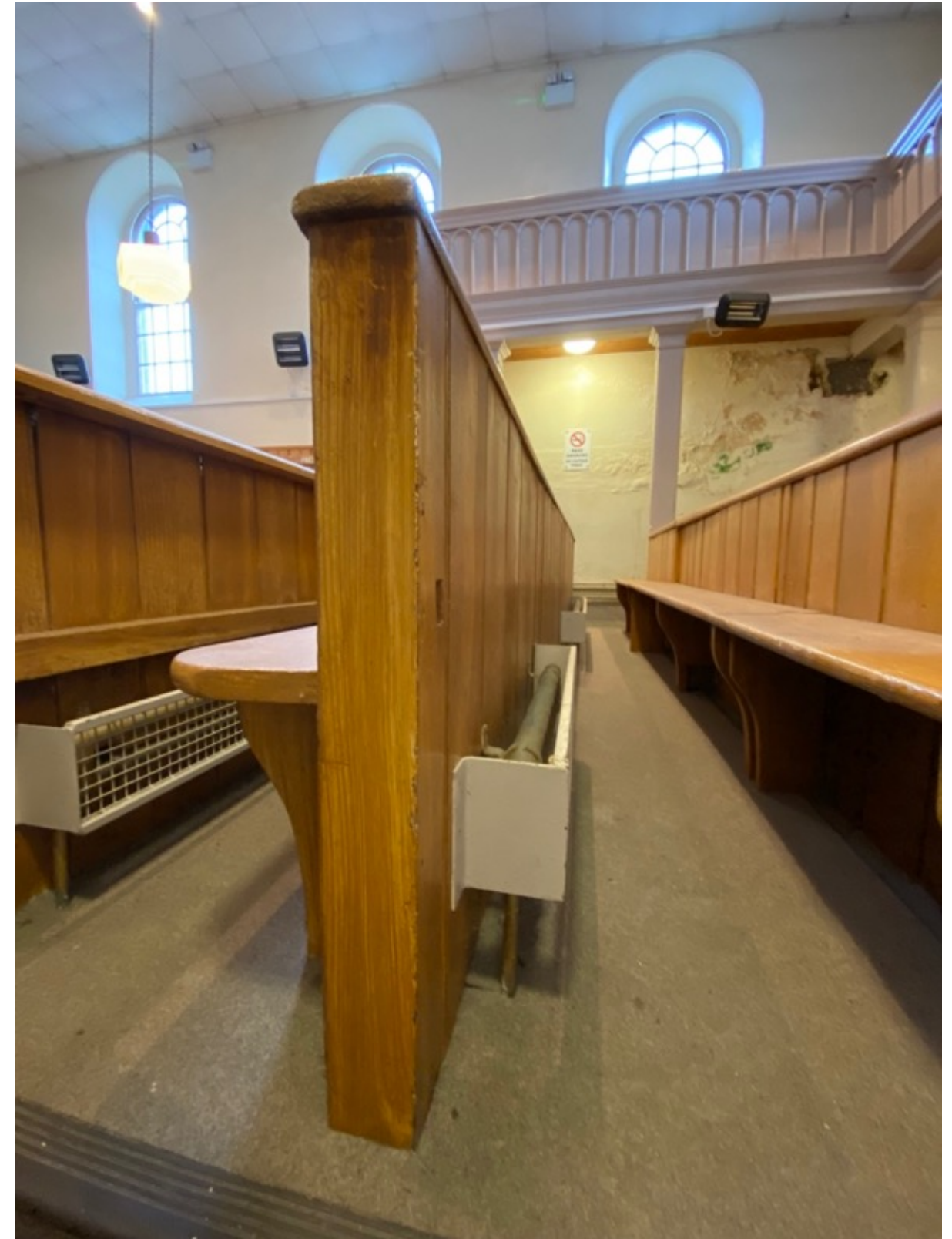
G05 – Courtroom – heating system
