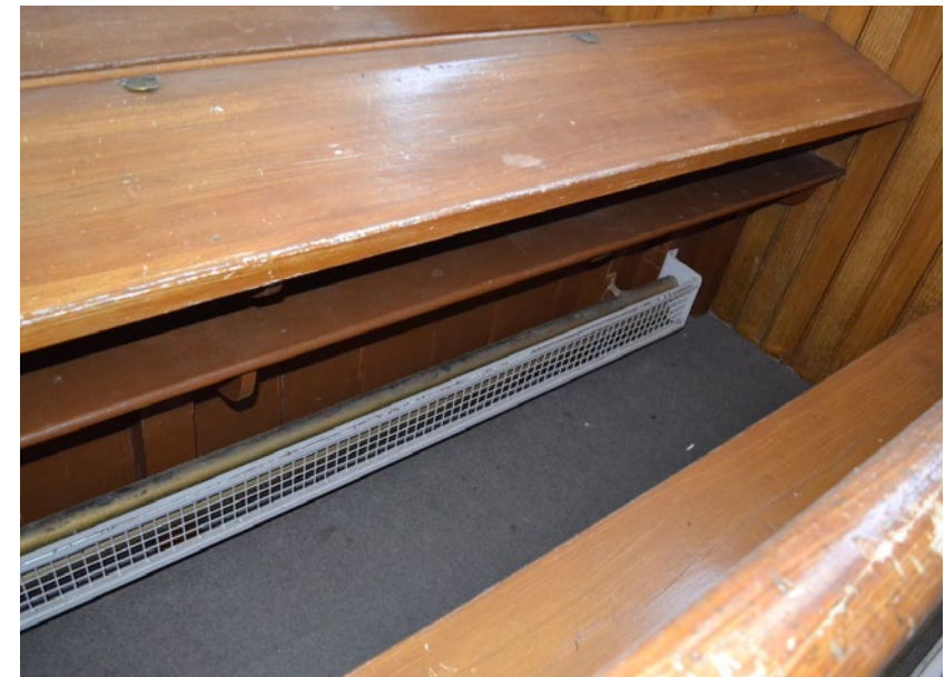
Figure 35 - Heating in courtroom
