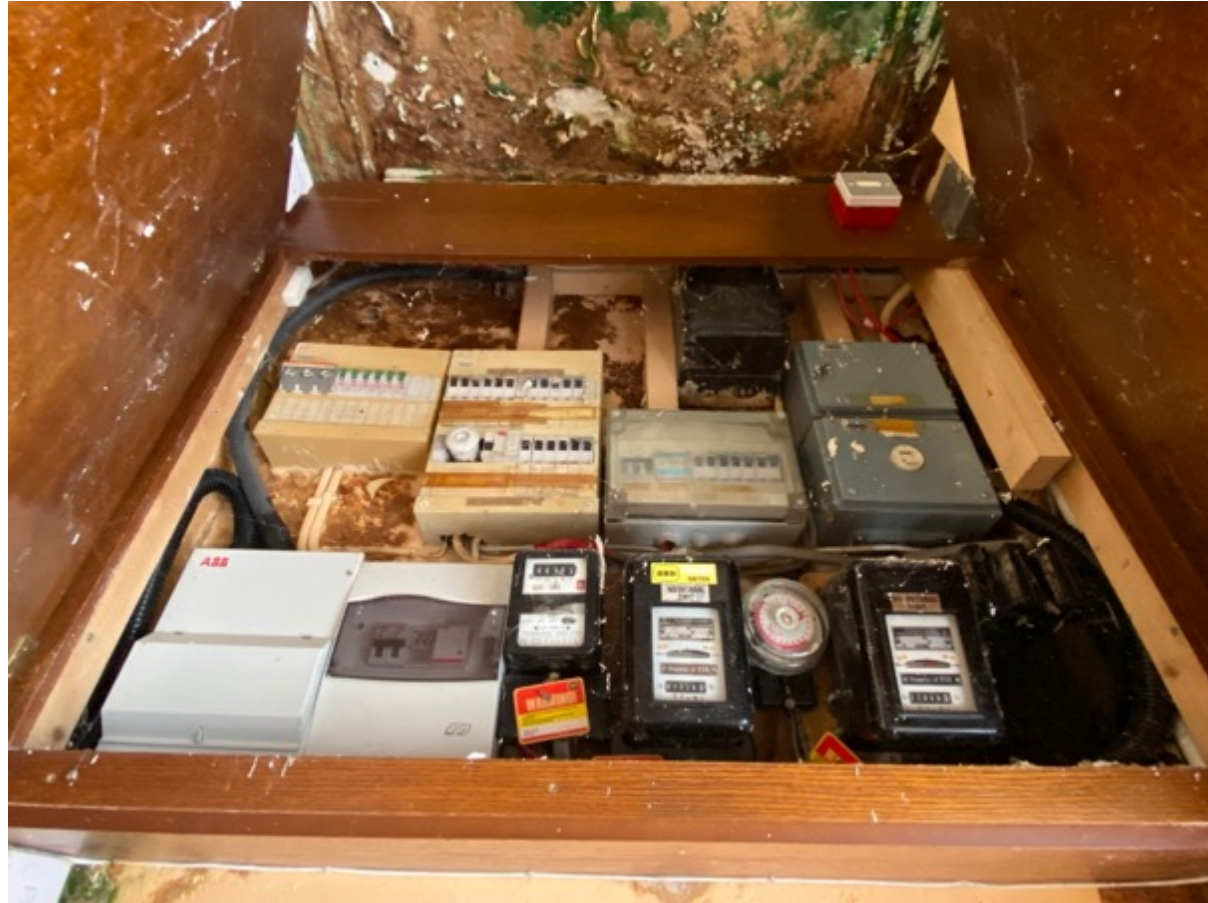
G02 - Reception - electrical panel
