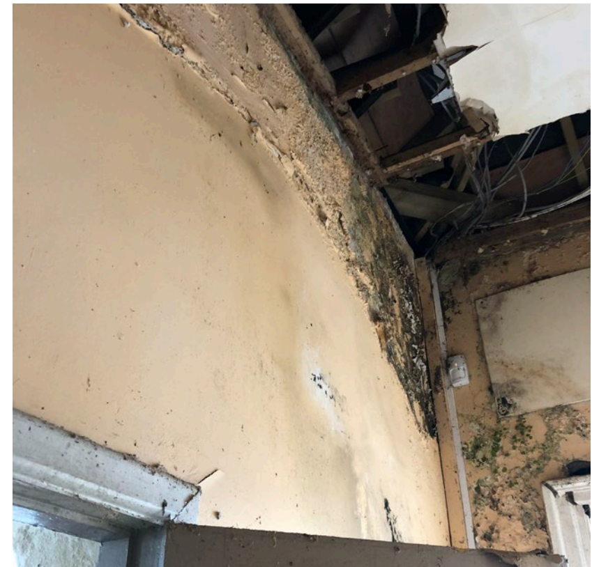
Figure 25 - Water ingress causing damage to the ceilings and walls
