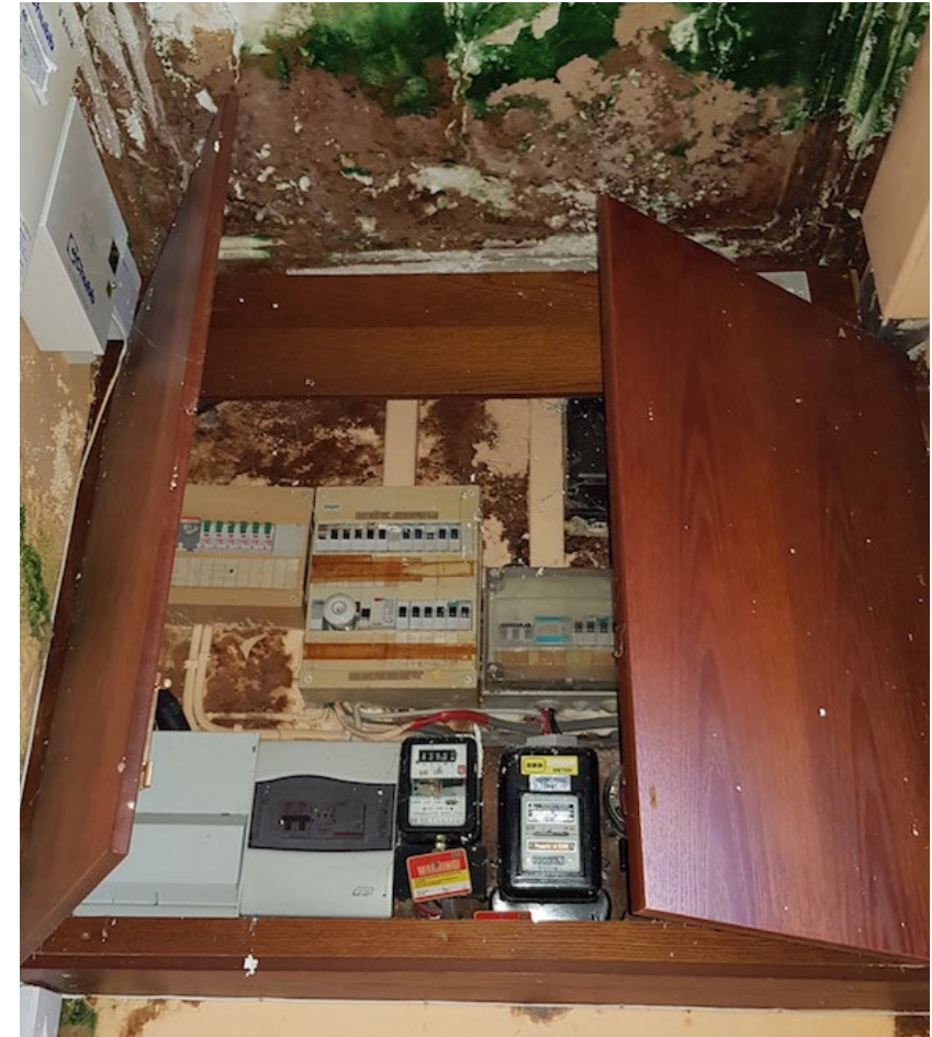
Figure 36 - Electrical box in ground floor entrance hall
