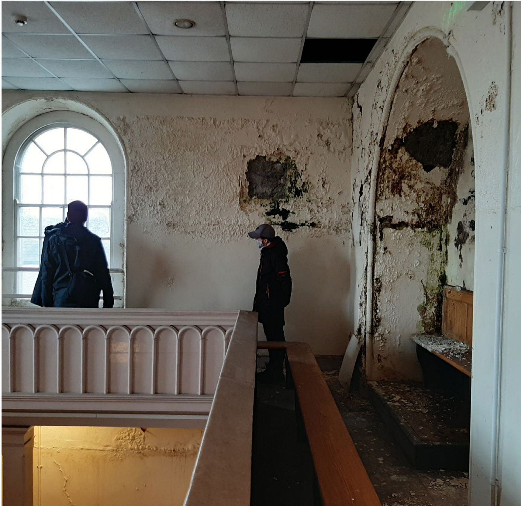
Figure 26 - View of the damaged plaster at gallery level of the courtroom
