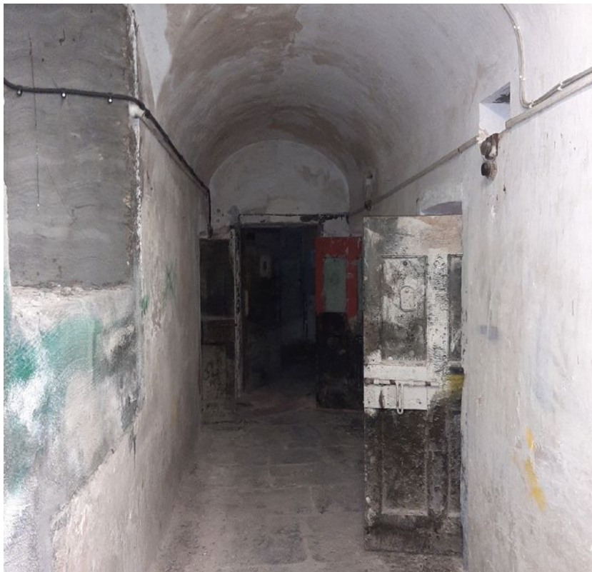
Figure 27 - View of the corridor in the cell block with original stone flags
