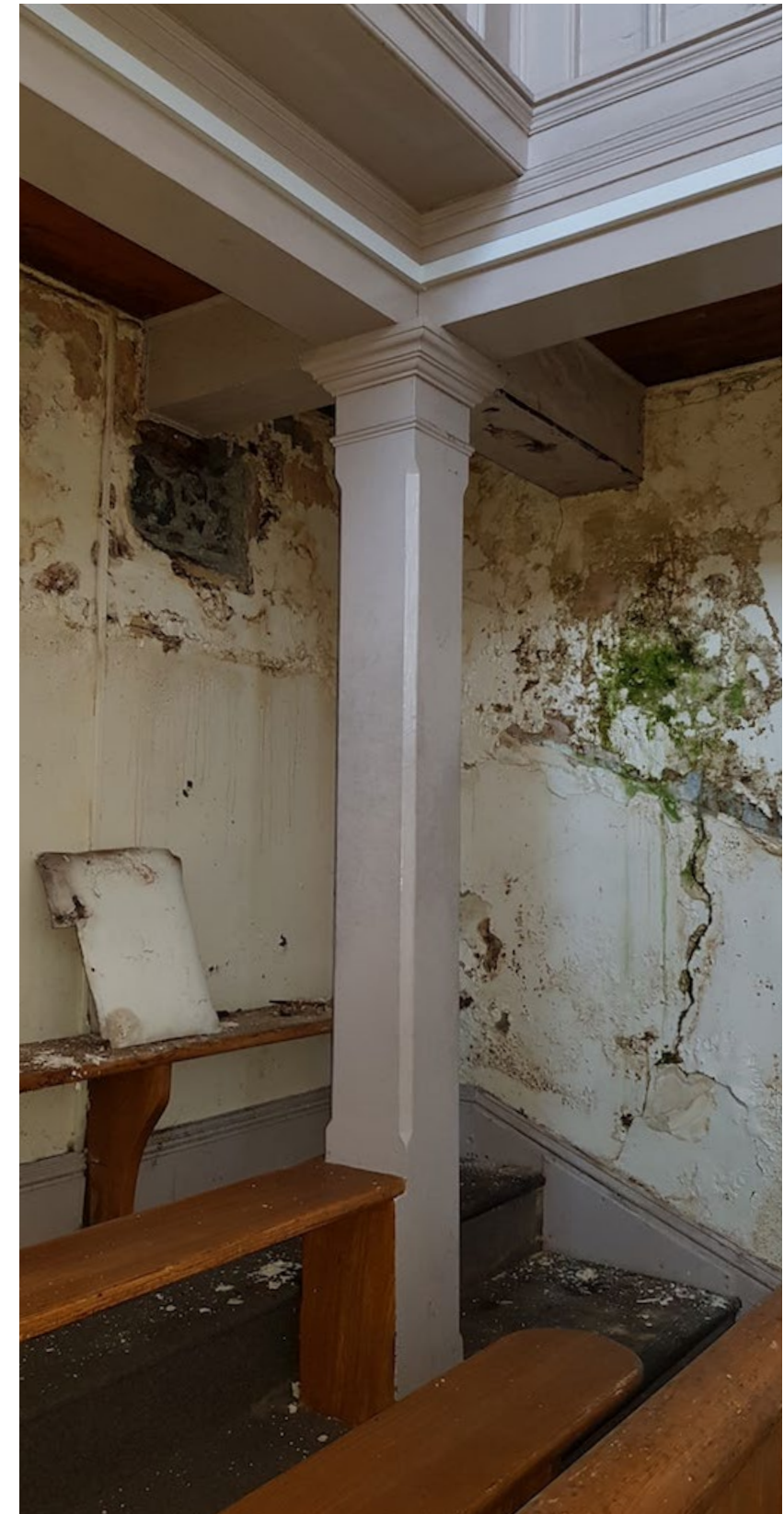
Figure 33 - Damage to plaster due to ongoing water ingress
