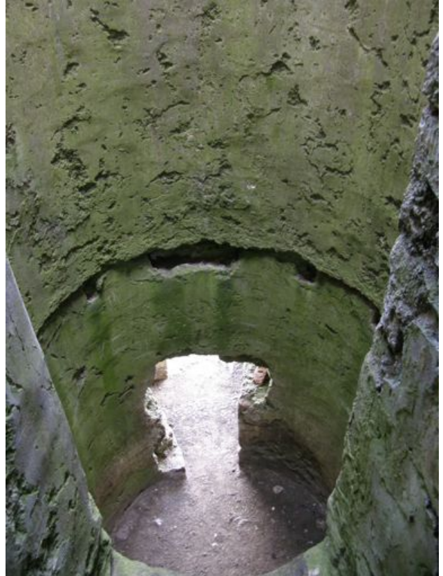
23 Inner drum looking downward to inner door ope
