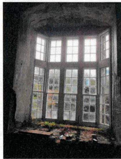
Photo 4 Water ingress above window
