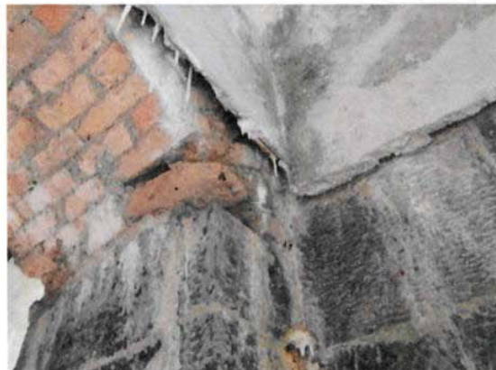
Photo 6 Lime Leaching Internal Walls
