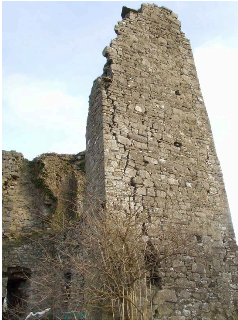
Structural cracking and voids west wall on line of patching of masonry
