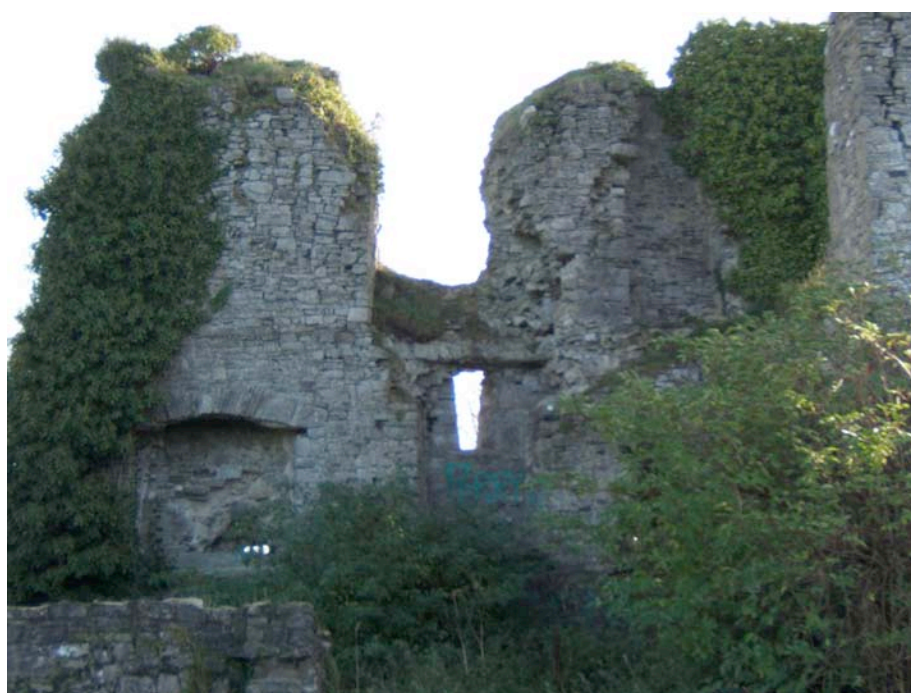
Extent of vegetation prior to cutting back - exterior south wall (top) and interior east wall (bottom)
