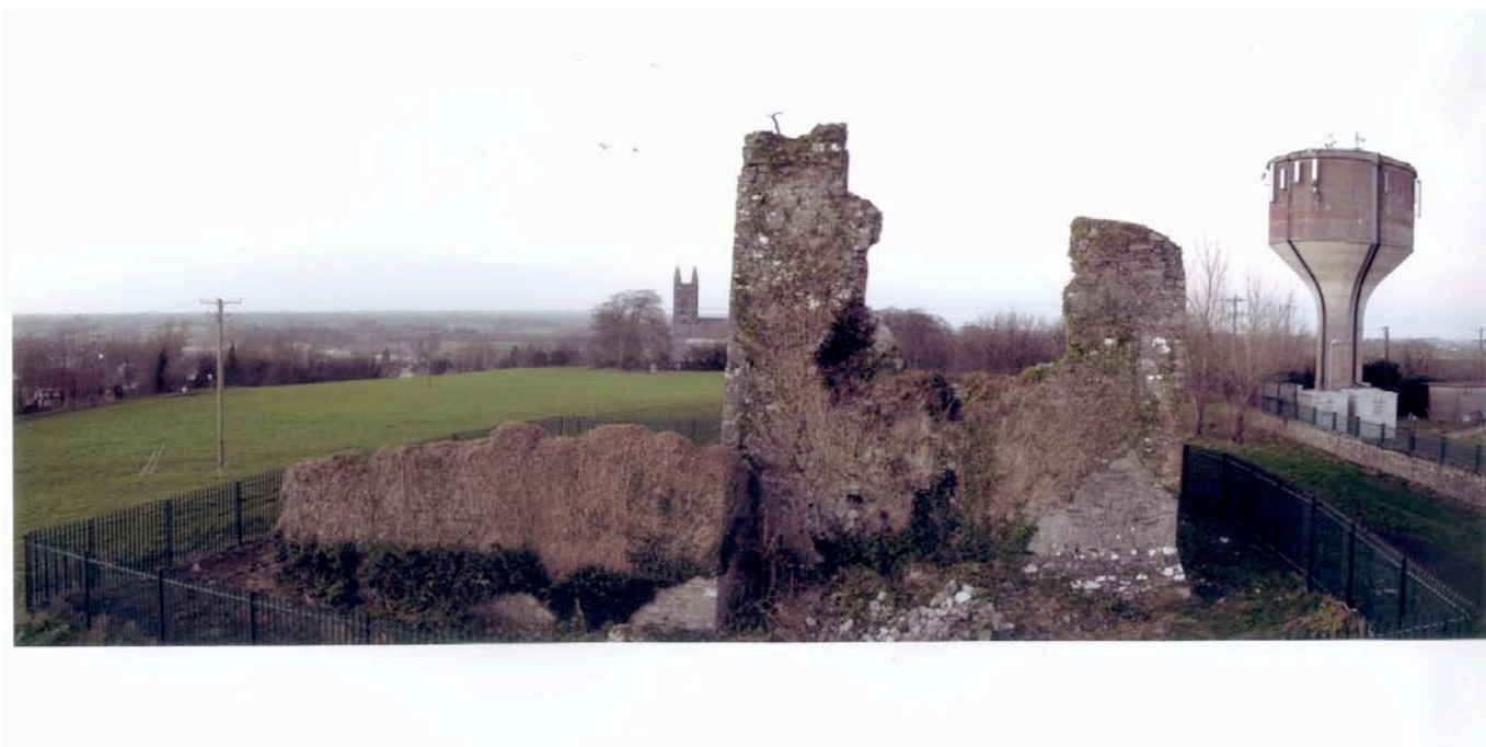
View from south with water tower and enclosure to the east and Church of Ireland in background. Note rubble from collapsed section of south wall
