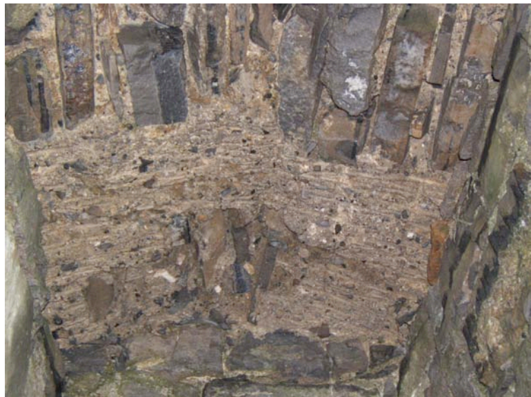
Traces of wickerwork centering still in place on head of opening east wall
