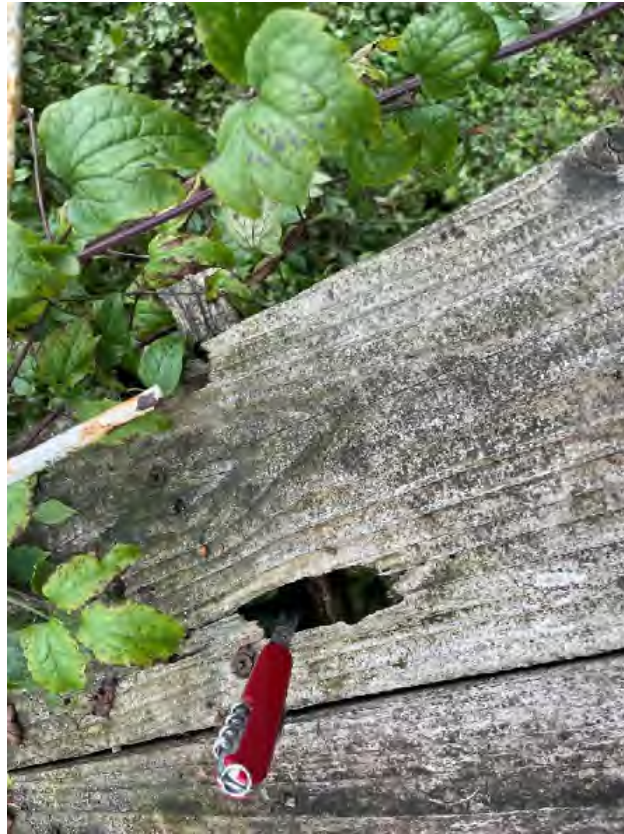
Timber in Poor Condition
