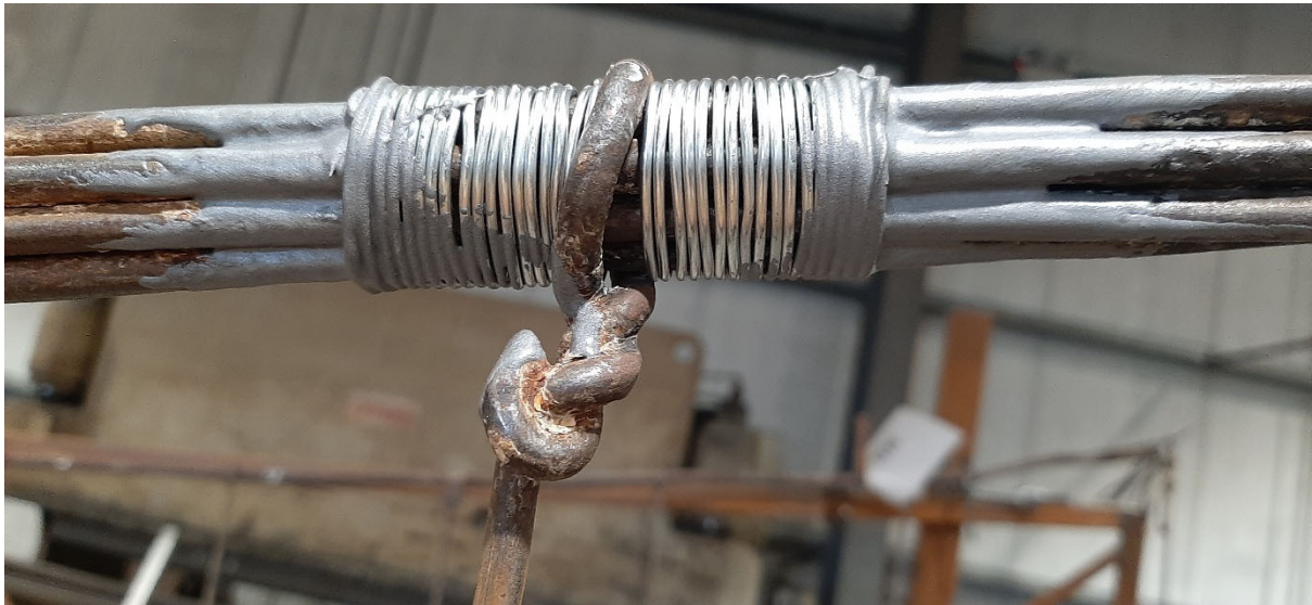
New binding wire under existing metal twists, to prevent future wearing through movement
